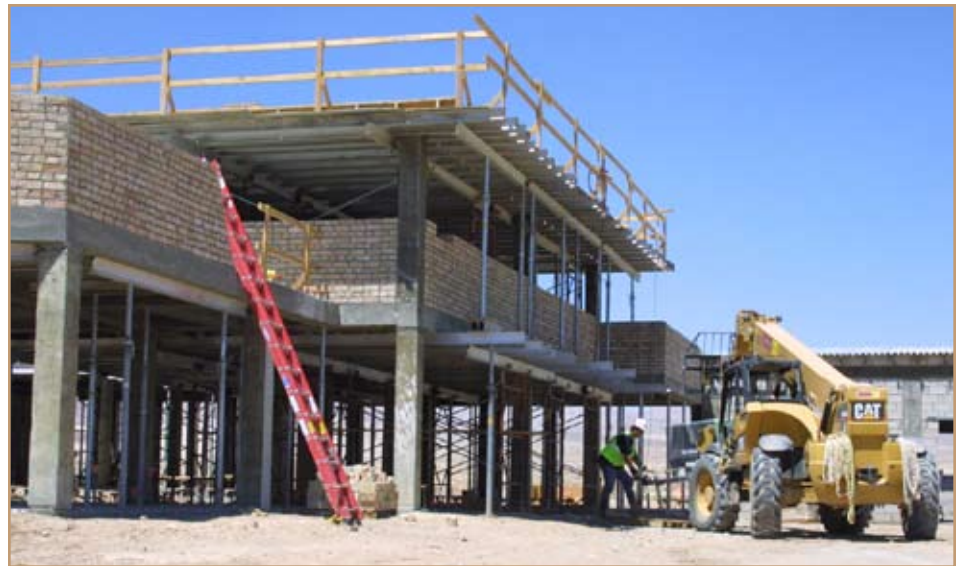
Contractors build up the outer walls of a simulated Iraqi village on Fort Irwin, Calif. The village was designed and built to Iraqi standards, except supports, which were built to withstand the seismic activity in the area. Photo by Daniel J. Calderón
