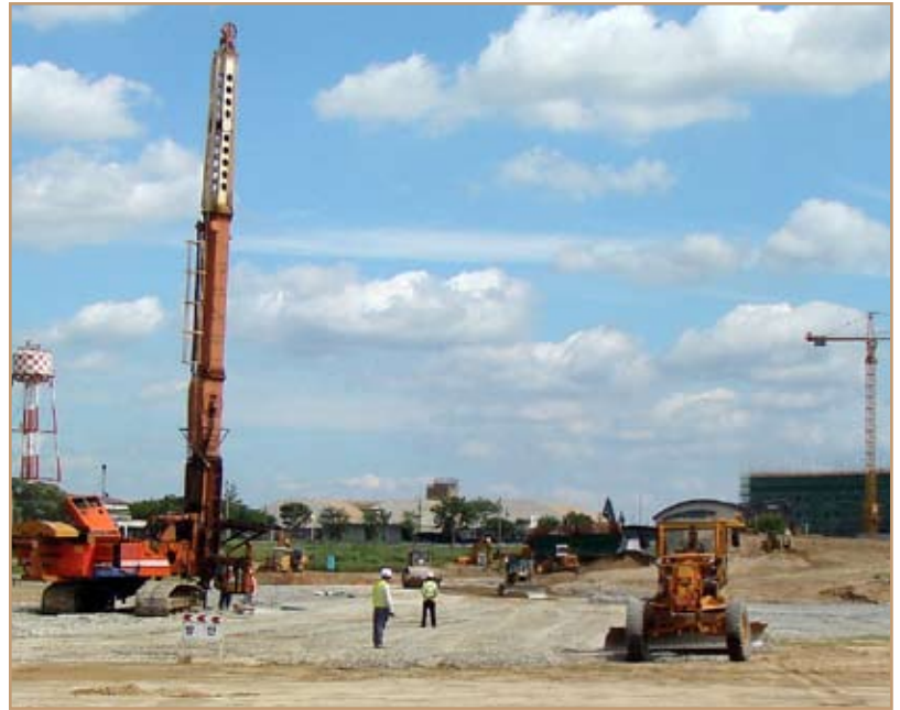
Far East District employees and local Korean contractors fill and compress new soil at Parcel 1, USAG Humphreys. Photo courtesy of USAG Humphreys
