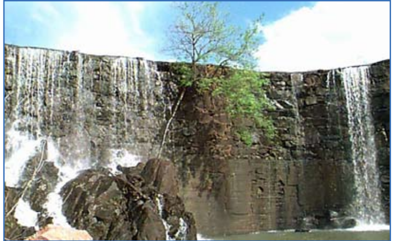
A tree grows out of the face of an Army dam, one of the factors that make it a high-hazard dam. Photo by Mike Dean
