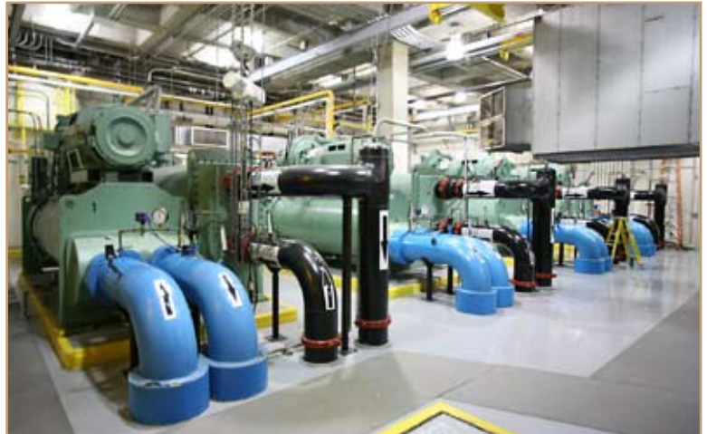
The use of corrosion resistant materials, high performance coatings and cathodic protection can prevent failures on systems such as chillers. Photo by Susan Drozdz
