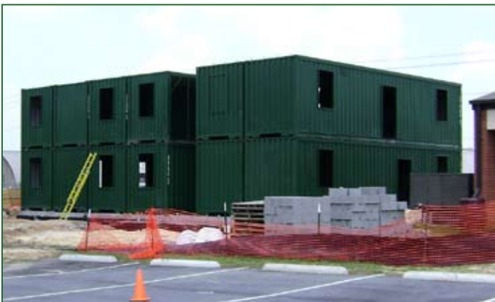
Fort Bragg's container building comprises 12 used 14-gauge steel shipping containers, each of which measures 9 feet 6 inches high by 8 feet wide by 40 feet long and weighs about 8,500 pounds. Photos by Erin McDermott.
