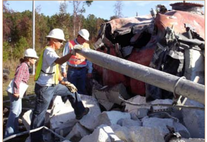
Amber Martin (left), Directed Demolition Service program manager for the U.S. Army Engineering and Support Center in Huntsville, Ala.; Alan Berdall (center), GEM Technologies site manager and David von Kolnitz (right), with the Military Ocean Terminal Sunny Point, N.C., Department of Public Works, look inside a torn open fuel tank, one of four 10,000-gallon tanks removed at the first Directed Demolition Service project. Photo by Chris Gardner
