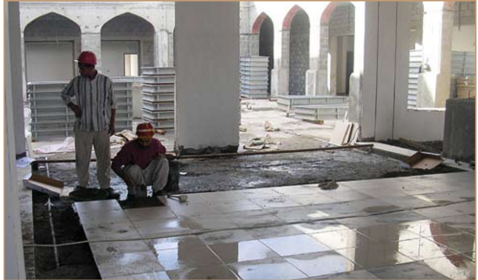
Workers at the Basrah Children's Hospital project lay down ceramic tiles. Some 800 people are employed by the project, which is scheduled to be complete by July. Photo by Betsy Weiner
