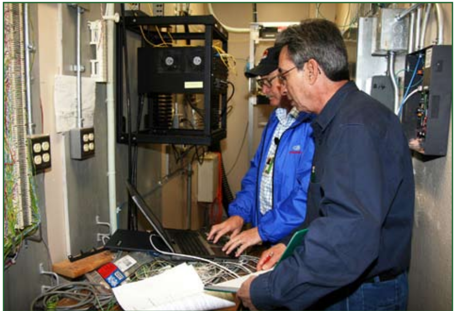
EMCS field supervisor Mickey Livingston (left), trains instrument technician Johnnie Silas (right), using a laptop computer to connect to the building controller. Photo by Michael Aident
