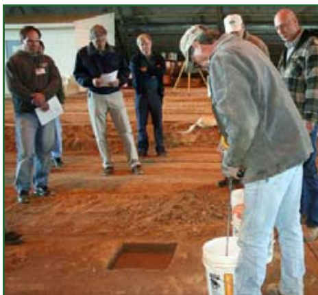
Students observe rapid pavement repair. Photo courtesy of the Engineer Research and Development Center
