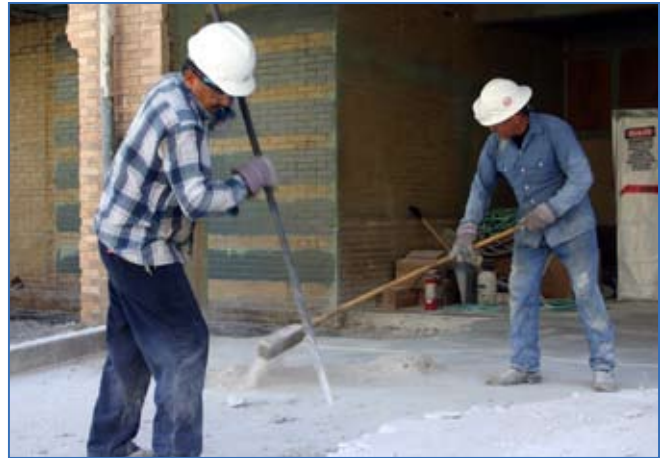
Gilbert Viera and Willie Garcia from RKJ Construction of Lampasas, Texas, remove concrete from the back of Building 2001. The building, along with adjacent Building 2000, will serve as the home of Installation Management Command, West Region. Photo by Elaine Wilson
