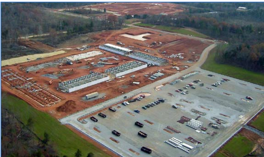
Barracks for the 2nd BCT are under construction in a historic district at Fort Campbell, Ky. Photo courtesy of Fort Campbell DPW
