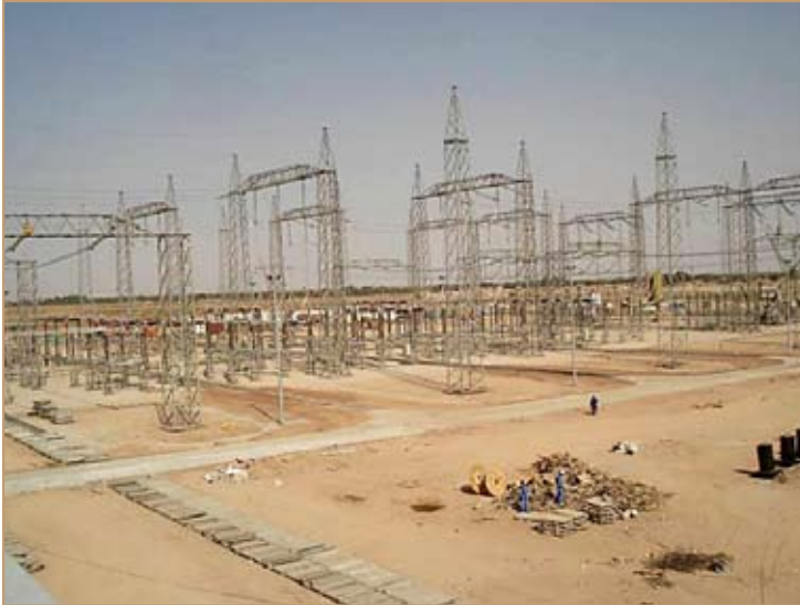
The Al-Amarah substation outdoor switchyard is where all the circuits come together and split to different directions in the country. USACE photo
