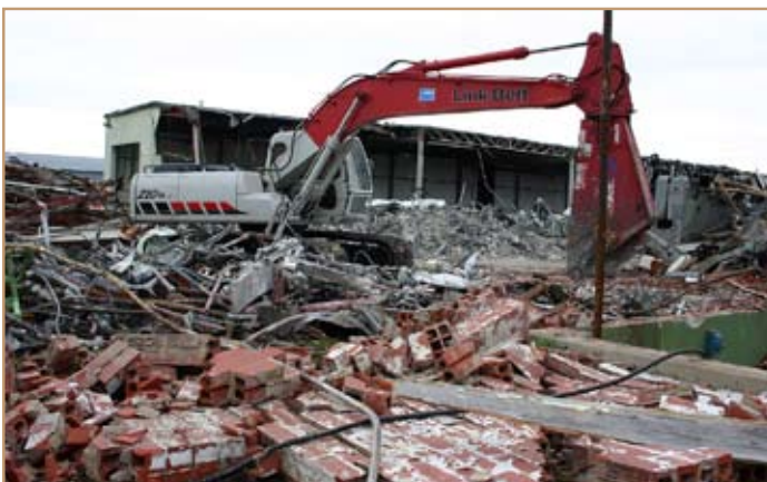
Contractors with Bhate Associates, Birmingham, Ala., will sort through this metal and brick debris to get materials ready for recycling.
