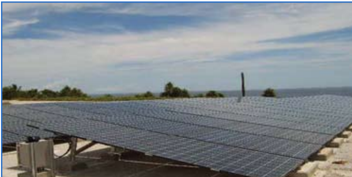
Photovoltaic panels in use on Kwajalein Atoll. Photo from the Army Energy Program web site
