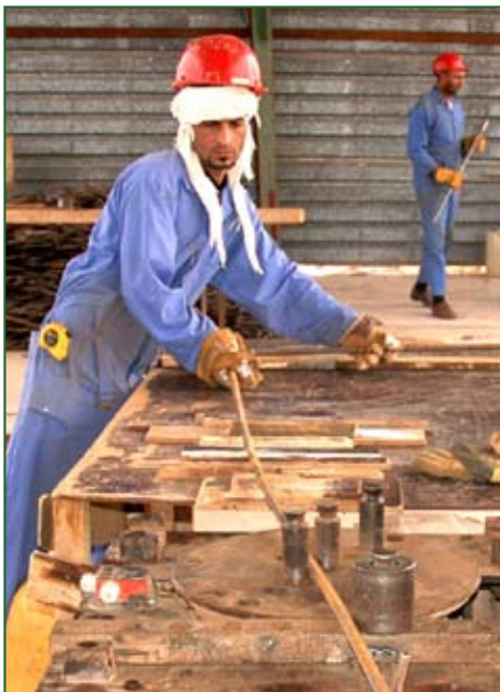
An Iraqi worker bends rebar for 12-meter-wide inlet tanks at Fallujah's new wastewater treatment plant.
