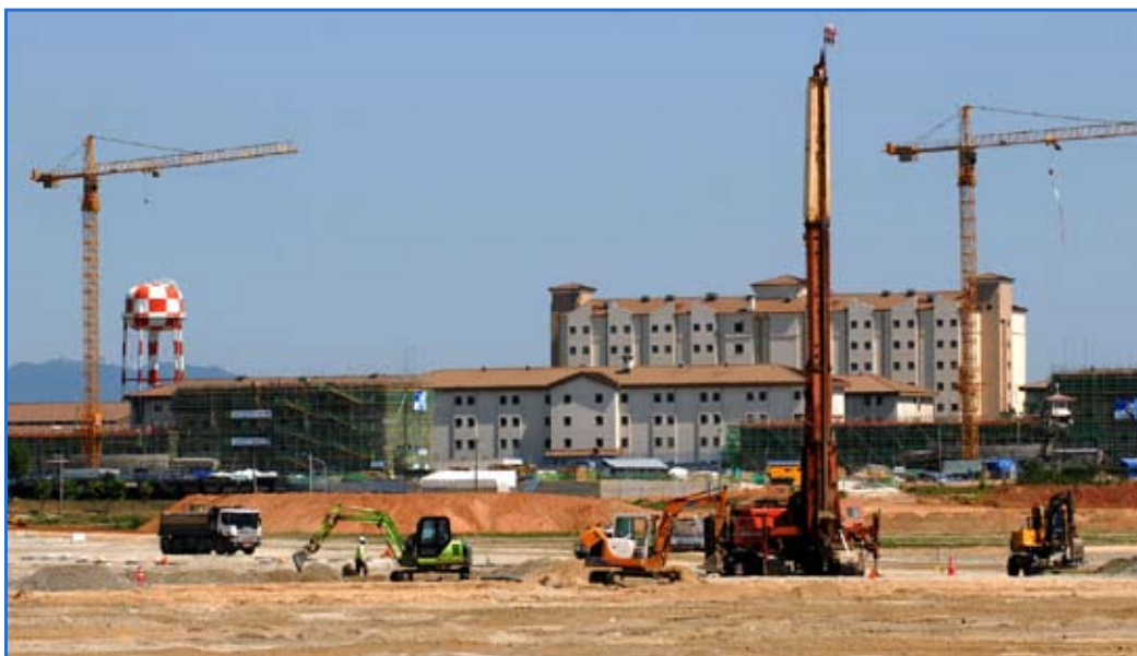
Contractors fill in what used to be rice paddies at U.S. Army Garrison Humphreys, South Korea. In the background, new barracks are being built on a site that a decade ago was a tent city used during training.
