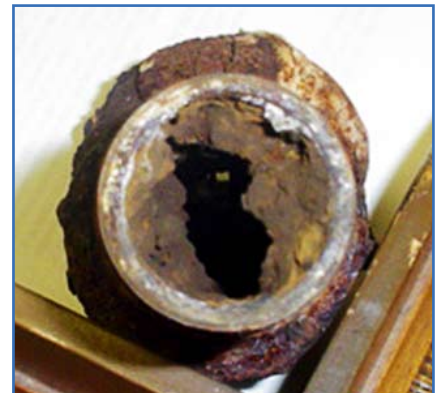
A portion of pipe removed for physical examination at Fort Benning, Ga., is severely occluded. Photos by David Miller
