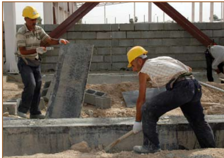
Workers set up for the foundation of the kitchen area for the new dining facility in Tikrit, Iraq. Photo by Lana Aziz, U.S. Army Corps of Engineers, Gulf Region North District
