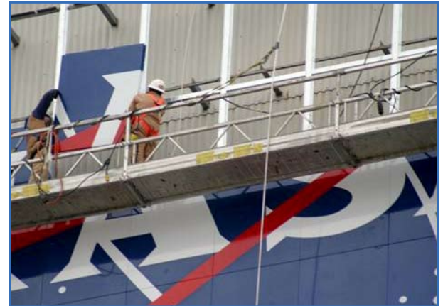
On scaffolds suspended from the top of the 20-story-high Vehicle Assembly Building, National Panel Systems’ workers Ken Harris and Patrick Chiles painstakingly place individual tiles of the NASA logo. Photos courtesy of the Engineering and Support Center, Huntsville, Ala.
