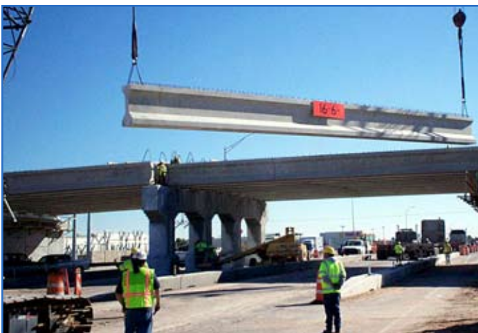
Work crews raise one of 20 pre-cast bridge beams. Each weighs more than 26.6 tons and is 65-foot long. Photo by Master Sgt. David J. Breitbach
