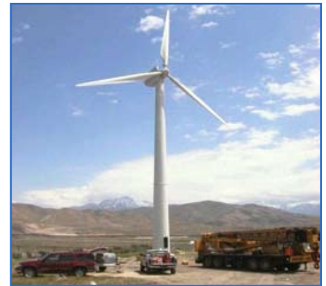
Wind turbines at Camp William, Utah, produce nearly one megawatt of electricity at full capacity. To comply with Executive Order 13423, the Army must increase use of renewable power sources. Photo courtesy of the Office of the Assistant Chief of Staff for Installation Management
