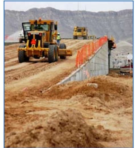
Crews process and mix ramp embankment material on site while using a grader, a scraper and vibratory compactors to pack together large areas. Photo by Edward Rivera
