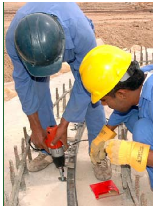
Iraqi crews work on the 12-meter-wide inlet tanks at Fallujah's new wastewater treatment plant. Photos by Norris Jones
