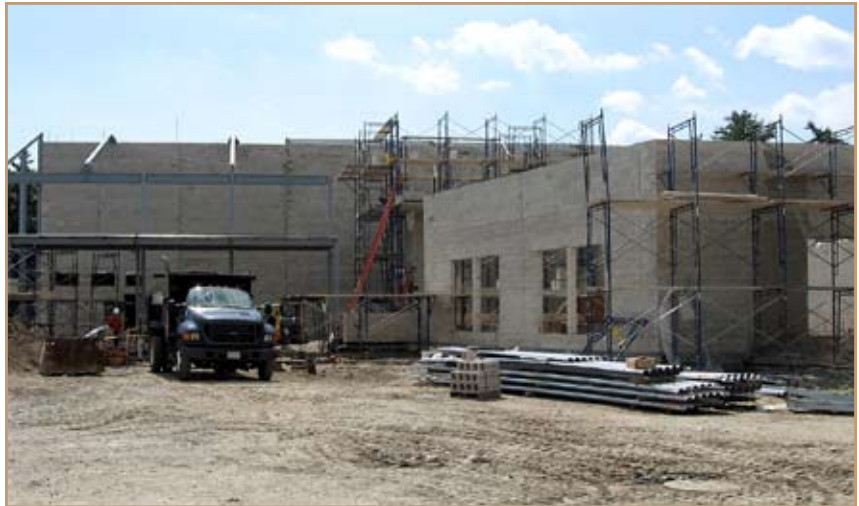
Construction of the new Hanscom Air Force Base fitness center is underway. Photo by Ken Paton
