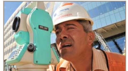
A contractor performs a precision survey for infrastructure planning for the high-tech campus.
