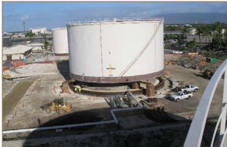
At Joint Base Pearl Harbor-Hickam, a fuel tank rests on stys so that new foundation ring walls and sand bedding can be installed underneath. Photo courtesy of Honolulu District, U.S. Army Corps of Engineers
