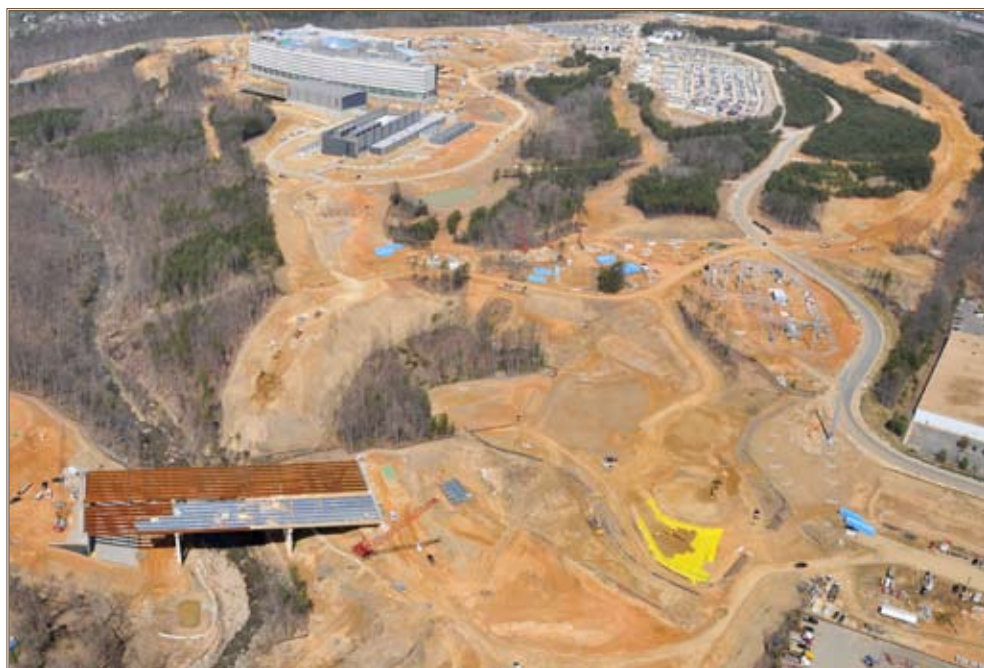
A single joint permit agreement covers road and storm-water management construction. Photos by Marc Barnes, U.S. Army Corps of Engineers
