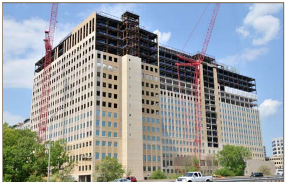
Precast exterior wall panels are quickly rising to the top of one of the office towers at the DoD Office Complex in Alexandria, Va. Photo by Marc Barnes, U.S. Army Corps of Engineers
