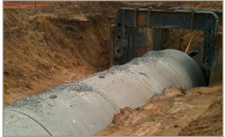
A storm sewer is repaired at Fort Benning, a project that used ARRA funds to improve infrastructure. Photo by Matthew Vera, Savannah District, USACE
