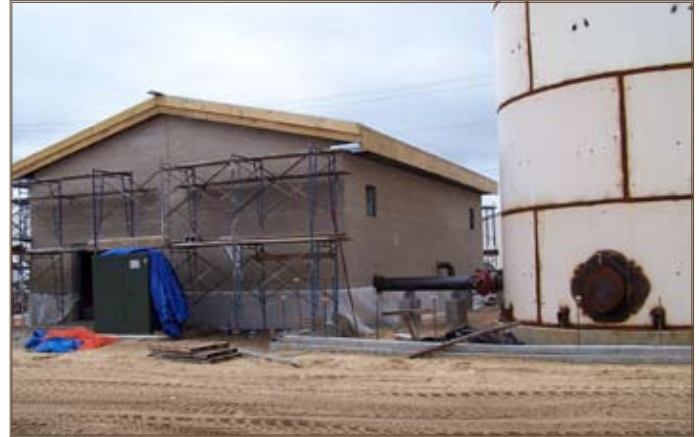
A pumphouse is under construction and water tanks are being refitted as part of the $5 million F-35 Infrastructure project at Eglin Air Force Base. Photo by Dale Smith
