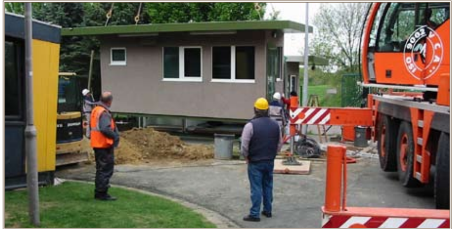
Workers install a new guard booth at Grafenwoehr Army Airfield, Germany, part of the ACP upgrades in Europe. Photo courtesy of Huntsville Center
