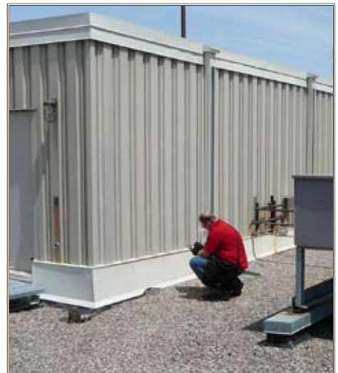
A contractor performs a roof inspections needed to implement ROOFER through an IDIQ contract managed by ERDC-CERL. Photo courtesy of ERDC
