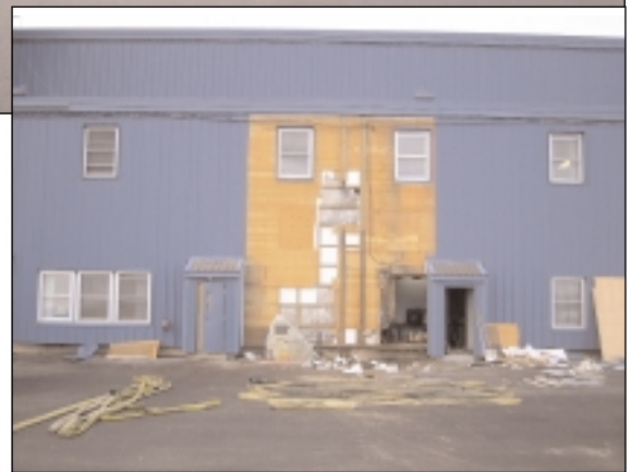
The exterior of the hangar showing the damage from the fire.
