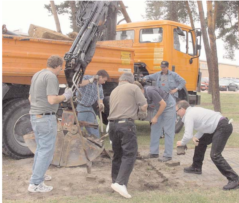
Team of DPW employees work together to remove an old concrete platform/foundation to enhance grass cutting and improve installation appearance on Taylor Barracks, Mannheim.
