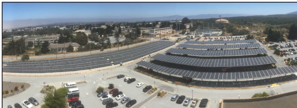
The completed 1-megawatt solar system at the Presidio of Monterey, California, combines ground and canopy mounted panels. (Photo by Jay Tulley)
