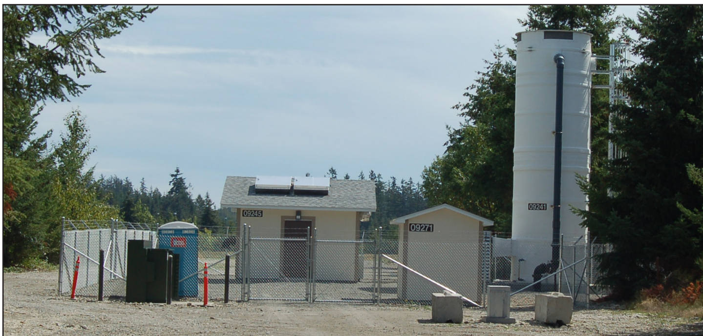
The Sea Level Aquifer Pump and Treat system at Joint Base Lewis-McChord, Washington, was repurposed to serve two critical needs on the installation, treating groundwater at the Logistic Center and meeting the water supply needs of the Madigan Army Medical Center's heating, ventilation and air conditioning system. (Photo by Tom Lynott)
