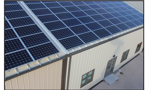
Fort Hood’s first Net Zero Energy facility is offsetting power needs with energy efficient technologies and a solar photovoltaic roof system, providing 91 percent of its electricity from renewable energy. (U.S. Army photo)
