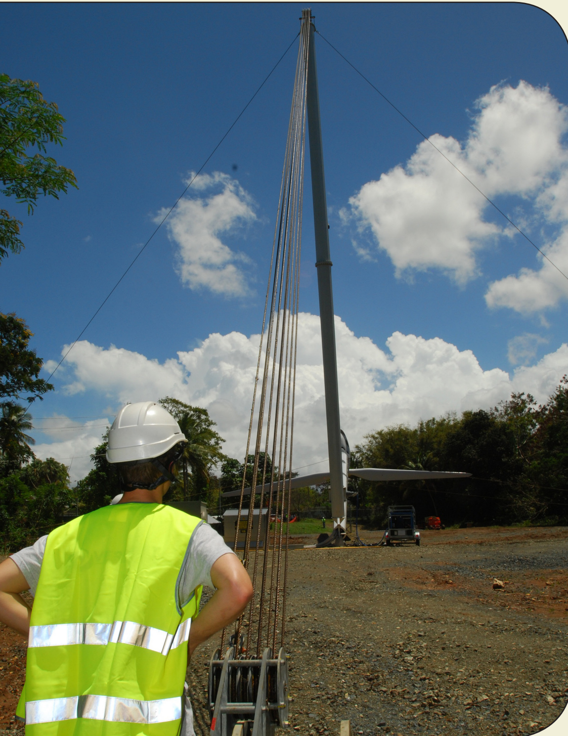
One of three 275-kilowatt wind turbines is installed at Fort Buchanan, Puerto Rico. The U.S. Army Engineering and Support Center, Huntsville, Alabama, awarded the $34 million task order. (Courtesy photo)
