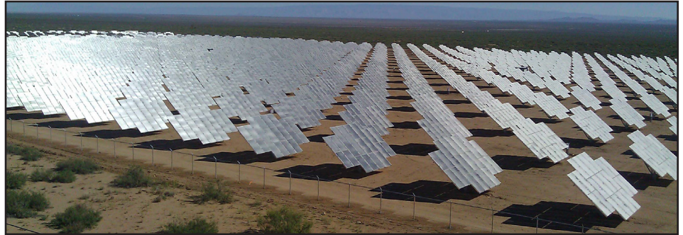
A bird's eye view shows the 42-acre solar array located at White Sands Missile Range, New Mexico, that is helping to save more than $2 million dollars in energy costs. It provides more than 4 megawatts of electricity to the installation. (Courtesy photo)
