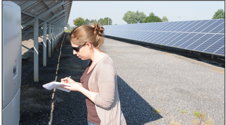
Mélanie Chaballe, energy manager, checks the solar panel inverters on Chièvres Air Base, Belgium. U.S. Army Garrison Benelux, Belgium, won the Secretary of the Army Energy and Water Management Awards small group category in renewables and alternatives for its Energy Conservation Investment Program 451-kilowatt solar panel array. (Photo by Donovan Abrassart)
