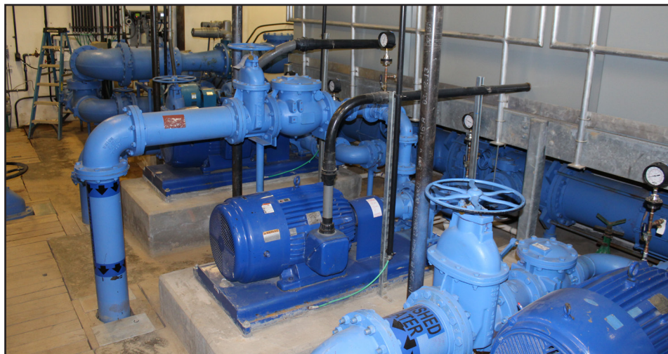
Massive pumps send finished water to the Fort Detrick, Maryland, garrison. The volume of water can be adjusted in minutes to meet increased demand. (Photo by Clem Gaines)
