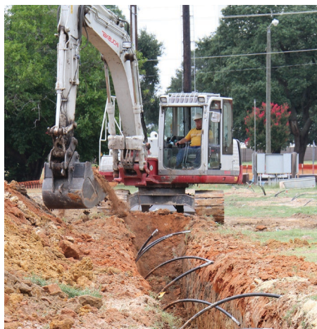
An excavator operator removes dirt from a trench in preparation for geothermal technology installation at Fort Bragg, North Carolina, Aug. 7. Photo by Elizabeth I. Gerhart.
