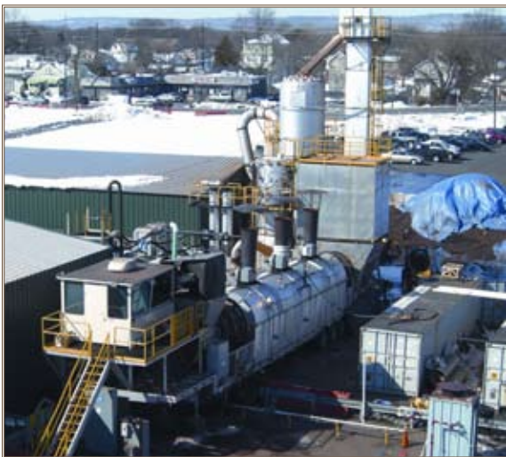
The low temperature thermal desorption unit at the Cornell-Dubilier Electronics site in South Plainfield, N.J., heats the soil, evaporating hazardous substances and converting them into solids that are disposed in a hazardous waste landfill. Courtesy photo
