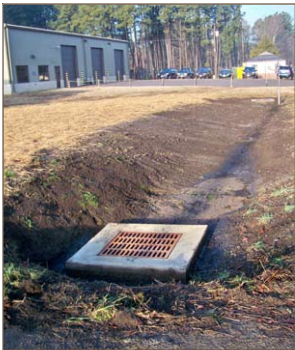
The design of a bioretention swale at a Fort Lee training area encourages maximum infiltration and reduced storm-water movement for other than extreme rain events. Photo by Dana Bradshaw
