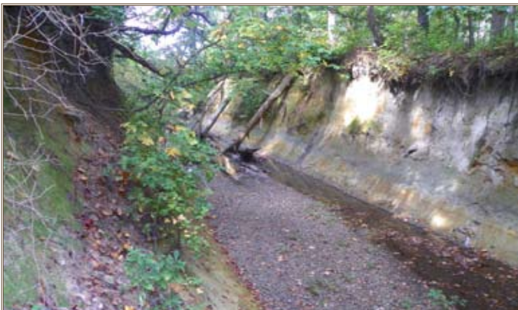
A heavily incised Bailey Creek tributary is more than 20 feet deep and 30 feet wide near the storm-water outfall. Photo by S. Nellis
