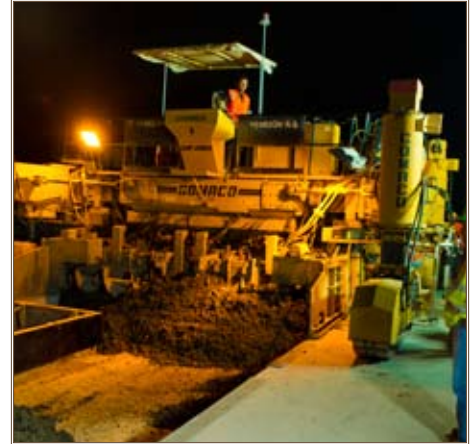
On Kandahar Airfield, a large paving machine places concrete at night so that the concrete does not have to cure in the heat of the day. Photo by Mark Ray, South District
