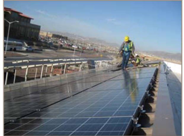
A worker strides along a row of solar panels installed atop a dining facility at Fort Bliss, a project that is part of a program that helps installations meet energy conservation goals.
