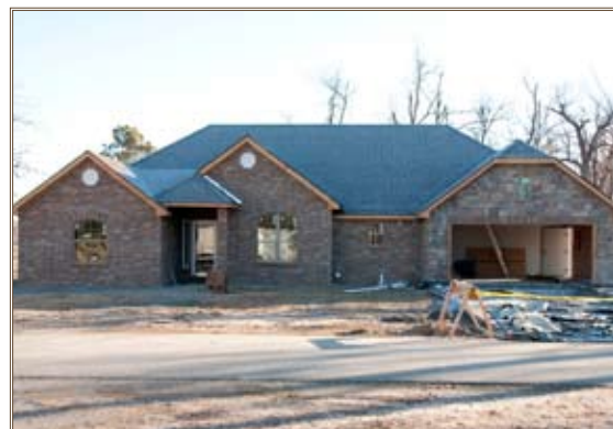
An American Recovery and Reinvestment Act-funded Family housing unit is under construction at Fort McAlester Army Ammunition Plant, Okla. Photo by Richard Smith, project manager
