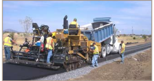
Workers build Fort Sill’s running and biking trail. Photo by Clarence Pierce III
