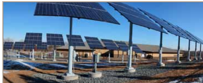
This photovoltaic array at the Arden Hills, Minn., Reserve Center is one of the Army Reserve’s projects to reduce energy use in a sustainable way. Photo courtesy of U.S. Army Corps of Engineers
