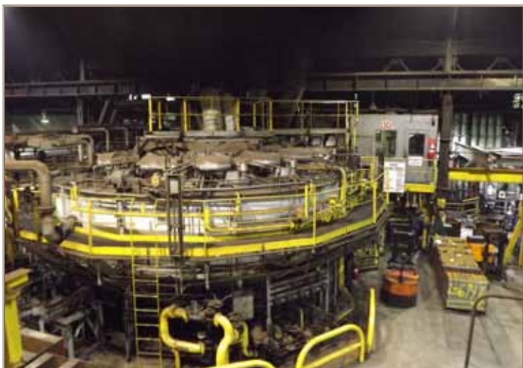
The rehabilitated Erie 1 Rotary Hearth Furnace's burners and heat recuperators reduce the furnace's natural gas consumption by 25 percent. Photo courtesy of SCAAP
