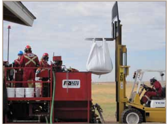
The contractor's field crew positions a super-sack containing micro-scale zero-valent iron and organic carbon above a mixing tank. Photo by Delma Stoner
