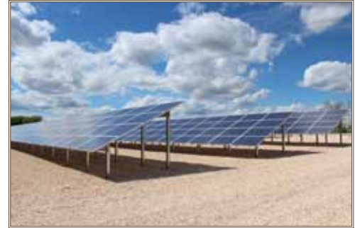
The solar panel field near Fort Hood’s Liberty Village consists of 3,000 photovoltaic panels on a four-acre site that generates one million kWh annually. Photo by Christine Luciano
