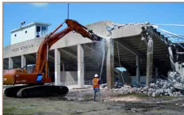
Contractors demolish the Prichard Sports Complex at Fort Hood, Texas. Photo courtesy of Charter Environmental
