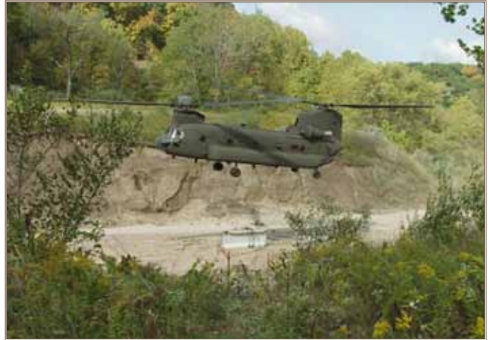
As part of an aviation training exercise, Illinois Guard Soldiers use helicopters to move concrete beams and place them in the stream. Photo by Jason P. McNamara, Marseilles Training Area
