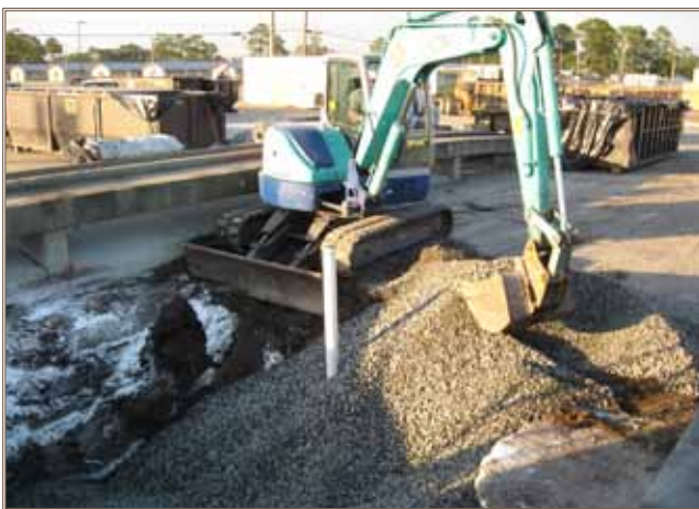
Soil contaminated by an underground storage tank is removed during construction of a tactical equipment shop and parking area as part of remediation efforts that also required treatment of the groundwater. Photos courtesy of FS-HAAF
