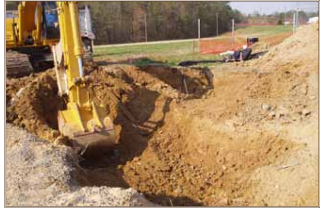
A backhoe removes explosives residue, petroleum hydrocarbon contamination and solid waste debris as an interim measure to streamline and accelerate the cleanup process at a Fort A.P. Hill former fire training pit site. Photo courtesy of FAPH
