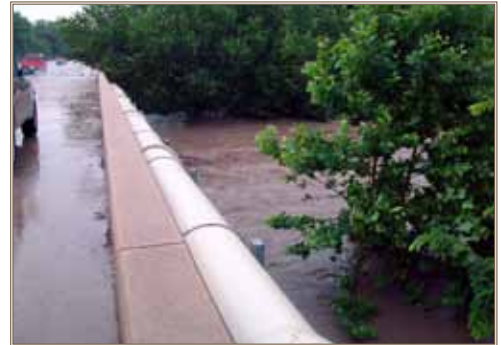
A flooded Wildcat Creek flows just under Scenic Drive near Fort Riley. Photo by Rob Ott, city engineer, Manhattan, Kan.
