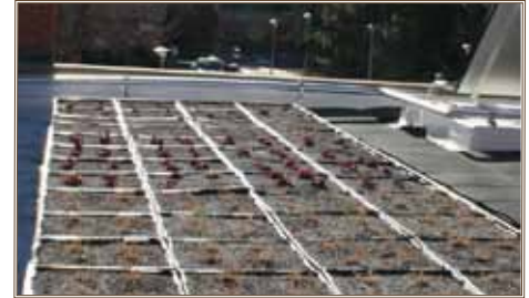
Data collected from Building 1219’s green roof will help determine Fort Carson’s best use of plants and grasses. Photo by Susan C. Galentine
