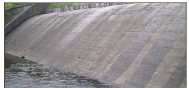
Stillwell Dam, a placed concrete structure, has a gallery at the base that allows inspectors to walk the entire length of the dam's interior. Photo by T. Coughlin
