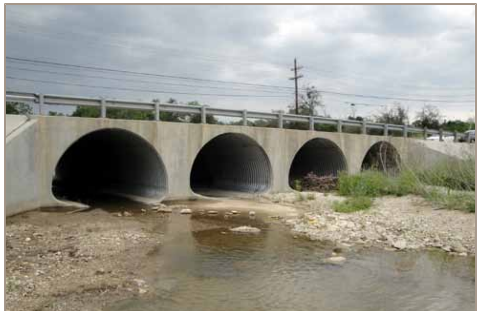
By law, bridges in the Army inventory, such as this Fort Hood, Texas, bridge, are inspected every two years. Photo by Gerardo Valazquez
