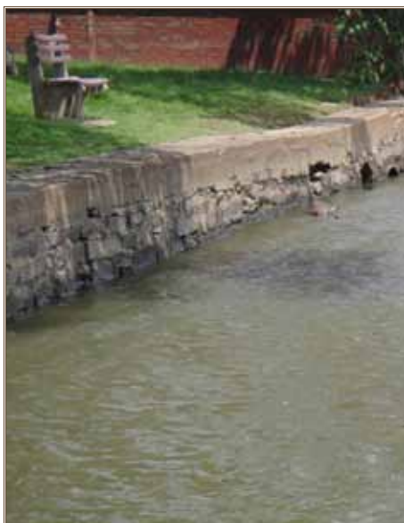
The Army's waterfront facilities, such as found at Fort McNair, Va., are inspected every four years by regulation. Photo by Kevin Haskins
