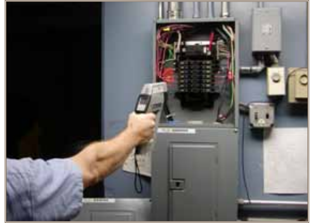
Fort Detrick uses infrared scanning to spot potential problems before they become serious. Photo courtesy of Fort Detrick
