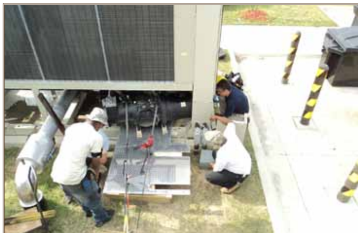
Air conditioning mechanics Nicholas Washington, Darrell Smith and Kevin Beekman replace a compressor on a barracks chiller at Fort Bragg. Photos courtesy of DPW, Fort Bragg
