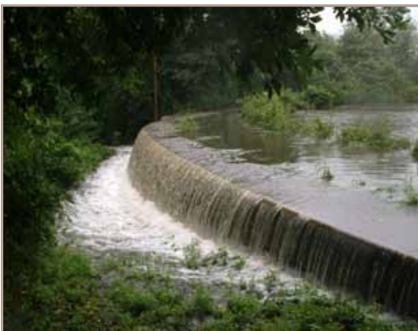
The 1846 Mine Lake Dam is topped during Tropical Storm Irene. Photo by T. Coughlin
