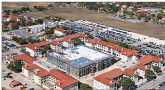
While a high performance IMCOM building at Fort Sam Houston, Texas, is under construction, two of the surrounding buildings (top left and bottom right) undergo major renovation to become HPBs. Photo courtesy of U.S. Army Corps of Engineers
