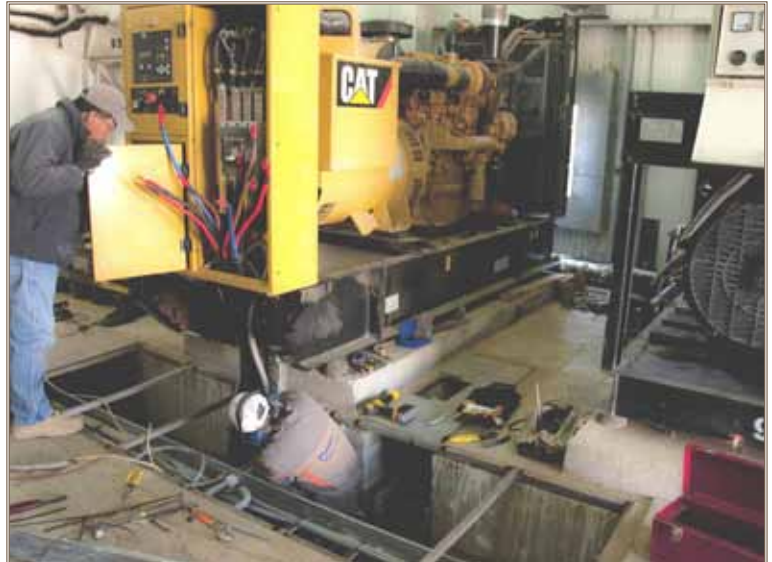
O&M workers install a new generator at the Joint Regional Afghan National Police Center, part of USACE efforts to ensure reliable power on the compound. Photo by Mark Ray
