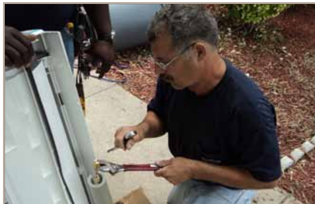
Air conditioning mechanic Bill Bradford prepares to install a ductless minisplit air conditioner on a Fort Bragg facility.
