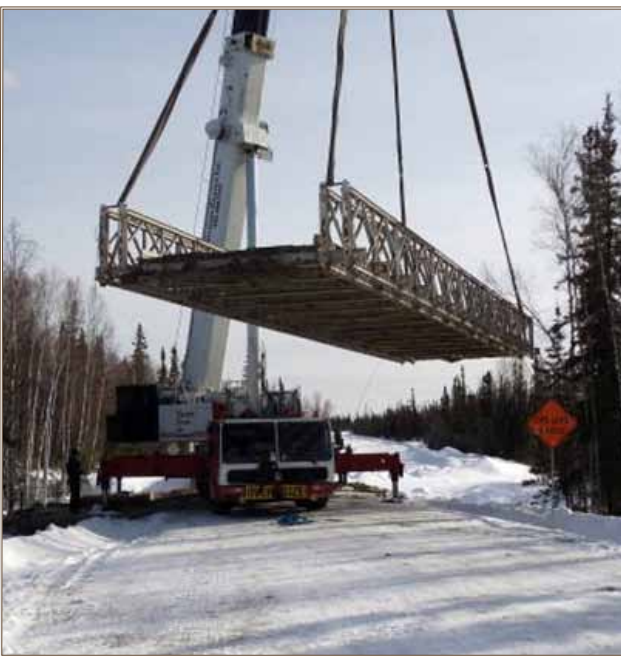
The Bailey bridge is lifted and moved to the roadway so that the cleaning and coating can be done away from the environmentally sensitive stream.
