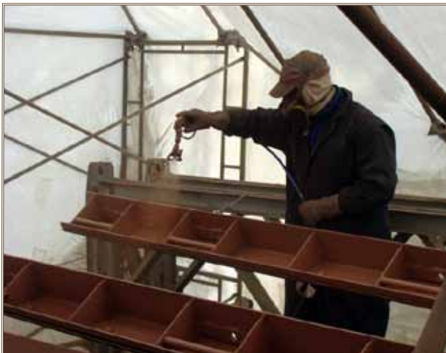
The low-VOC coating is applied in cold temperatures using airless spray. Photos courtesy of ERDC-CERL
