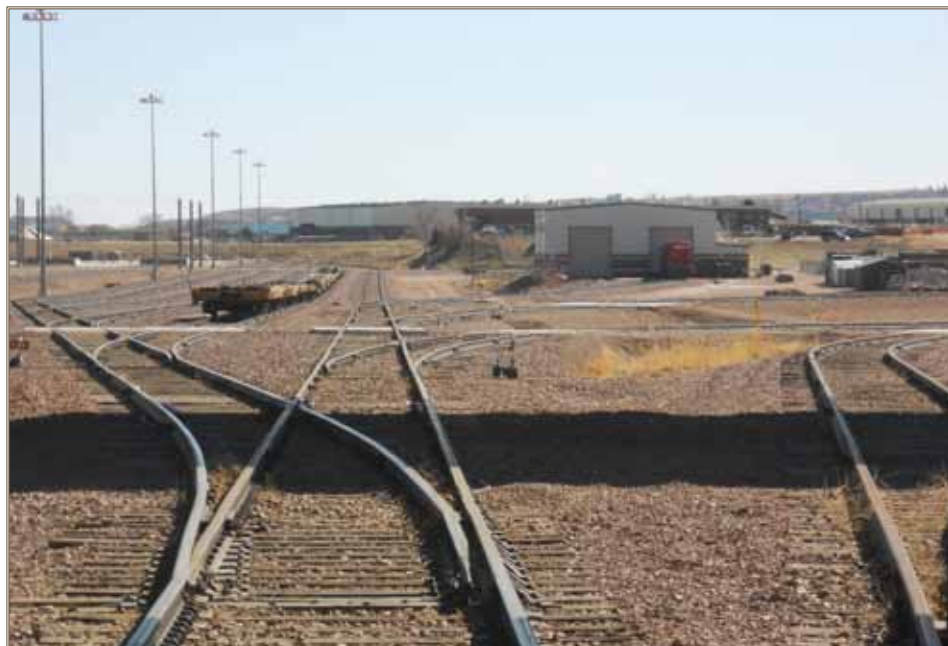
Railroad infrastructure, like these tracks at Fort Carson, Colo., is inspected every four years. Photo by Mike Crawford
