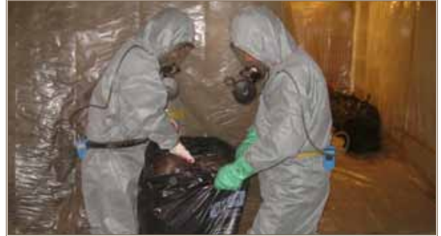
In-house Asbestos Removal Team members double bag asbestos debris in preparation for disposal at USAG Yongsan. Photo by Na Chong Pok
