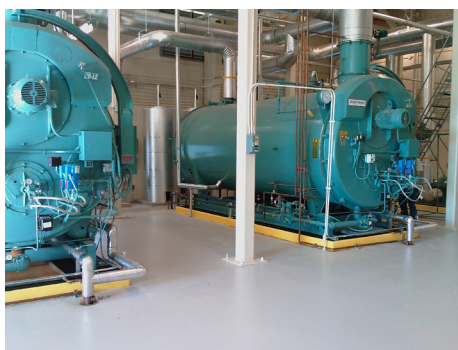
OMEE projects include industrial boilers and pumps.
