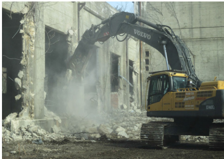
The Facilities Reduction Program removes excess facilities from installations, such as the heat plant shown here. (North American Dismantling Corp.)
