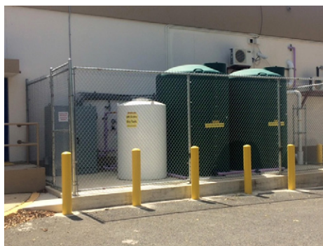
Tanks in place at building 606, PXtra store.
