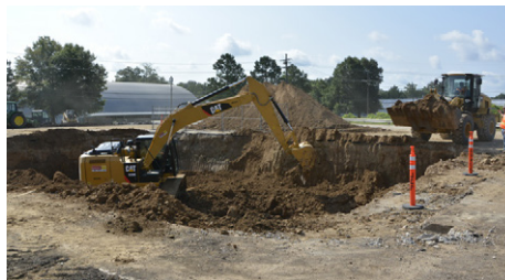
Twenty-five hundred cubic yards of soil were excavated, treated for contaminants and replaced.
