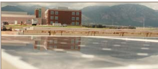
A 500,000-watt photovoltaic array system that will help bring Fort Carson nearer to its net-zero goals is under construction outside the 4th Brigade Combat Team, 4th Infantry Division’s new brigade and battalion headquarters building. Photo by Andrea Sutherland
