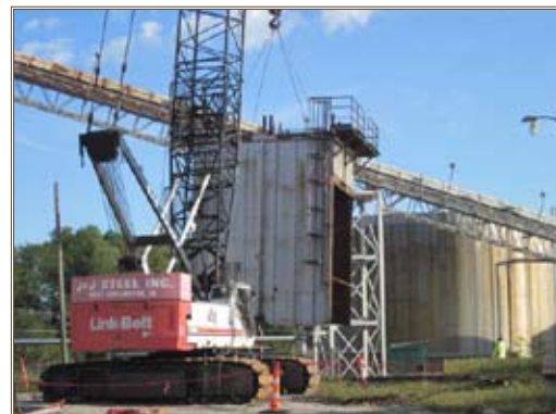
A crane removes the electrostatic precipitator from the main heating plant at IAAAP. Photo by Arthur Shattuck
