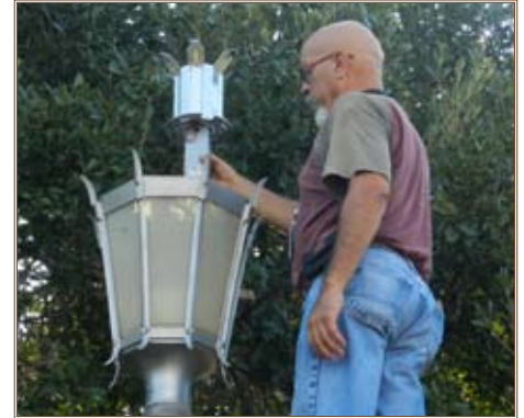
A worker installs an LED fixture in antique lamp post at Fort Sam Houston. Photo courtesy of Frank Thomas
