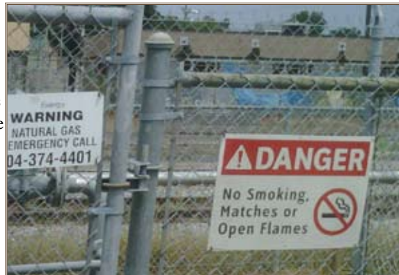
A gas meter behind a locked fence is inaccessible to a meter reader. Photo by Deborah Lamb-Boatwright
