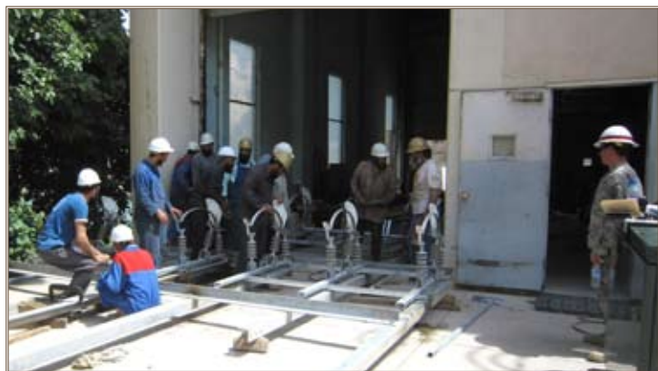
Sgt. Terry Dietrick (right) looks on as DABS engineers work to construct the switch center that will reduce the number of daily circuit interruptions at the Kajaki Dam. Photo by Chief Warrant Officer 5 Thomas B. Black
