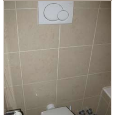
A Vicenza, Italy, barracks bathroom has dual-flush toilets, a “low-hanging fruit” water-conservation measure that many installations have already added. Photo courtesy CERL
