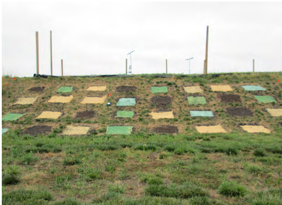
Svendsen - ErosionControlBlanket.jpg - Erosion control blankets protect a revegetated hilly area from runoff. (ERDC)
