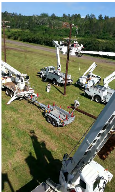
Company A, 249th Engineer Battalion (Prime Power), U.S. Army Corps of Engineers, completes joint training with the Directorate of Public Works, U.S. Army Garrison, Hawaii. (249th)
