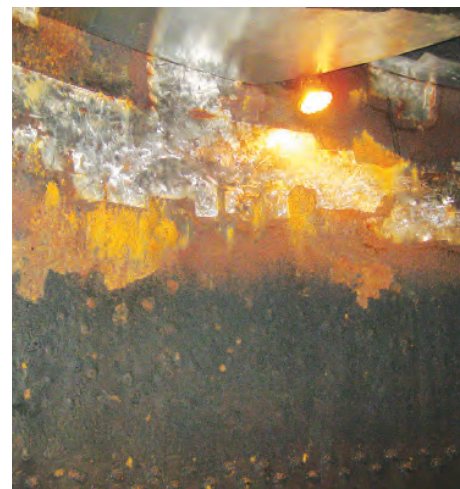
The shiny areas show where previous cavitation repairs have been made. The yellow areas show new areas of cavitation that will be repaired during this maintenance period.
