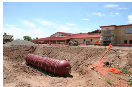
The 30 thousand gallon rainwater collection tank at the Reception Complex. (B. Purdum)
