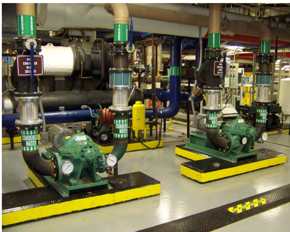
This is an example of pumps found in a mechanical room in a hospital. The Operations and Maintenance Engineering Enhancement Program maintains the facility and performs preventative maintenance and repairs to these type systems. (USACE)
