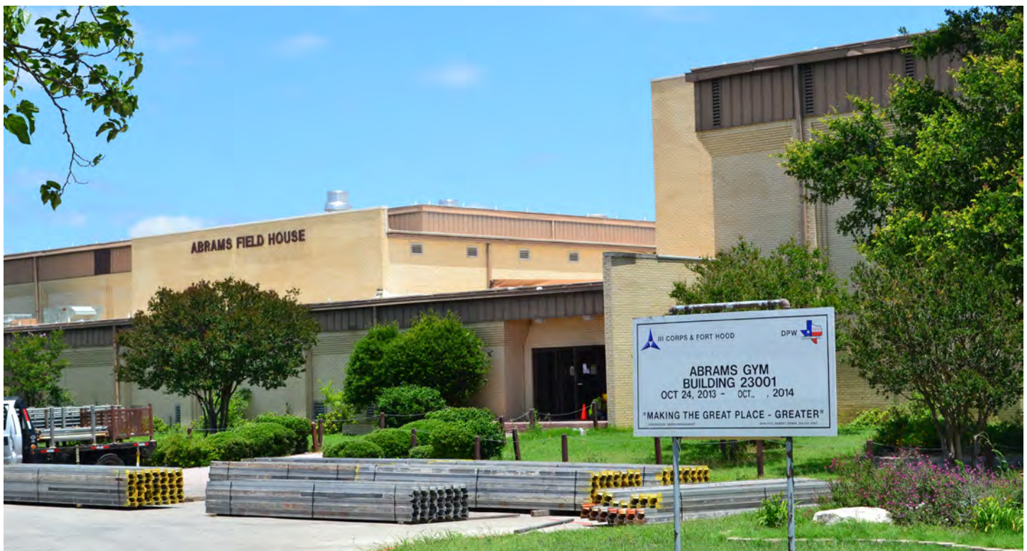
Ongoing renovations in Abrams Gym will providemodernized and efficient infrastructure for Soldiers and their Families. (CPL B. Sigola)
