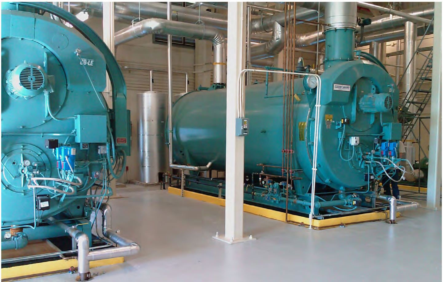
Other Operations and Maintenance Engineering Enhancement examples include boilers like those installed at Womack Army Medical Center at Fort Bragg, North Carolina. (R. Hilton)
