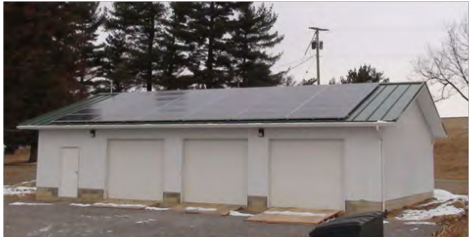
Photovoltaic solar panels installed on the roof of the maintenance shed at Beach City Lake in Beach City, Ohio.
