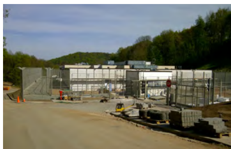
Work continued last November on the new U.S. Army Regional Correctional Facility-Europe at Sembach Kaserne, Germany. It's being built as a replacement for the corrections facility at Coleman Barracks in Mannheim. When completed this summer, the complex will house up to 40 individuals during pretrial and post-trial confinement, as well as sentence duration, with separate quarters for men and women.
