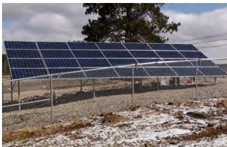
Ground mounted photovoltaic solar arrays like this is the type of installation location found at seven of the eight Huntington District lakes which will receive the solar panels.
