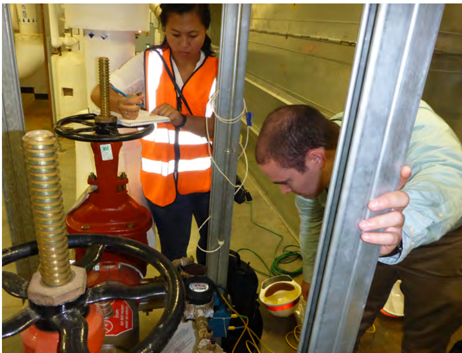
Civil engineers set up a flow recorder to on a barracks potable water supply at Fort Leonard Wood. (ERDC-CERL)
