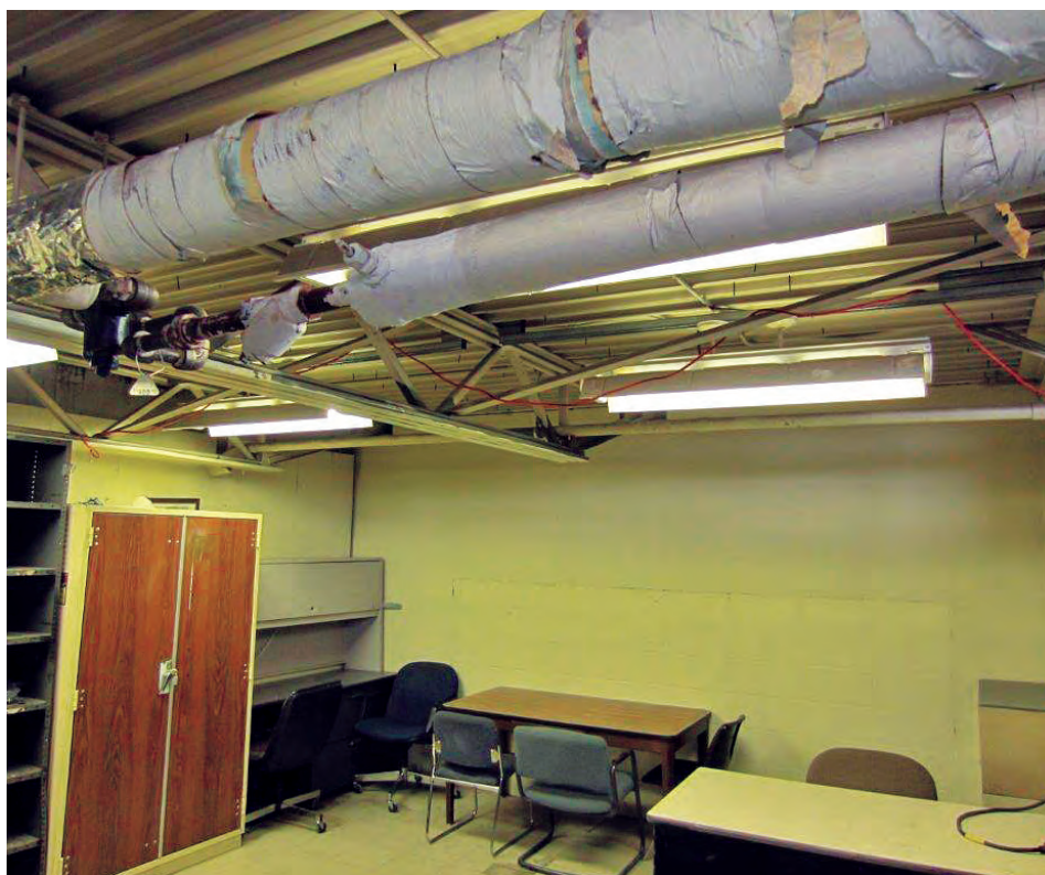
Maintenance shop with damaged/missing insulation on pipes, and an uninsulated ceiling
