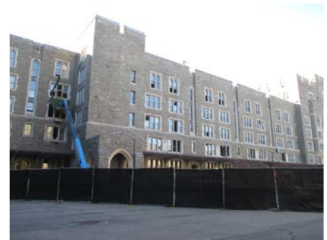
A glimpse of the North-South wing of Scott Barracks under construction (photo by Kenneth Stay)
