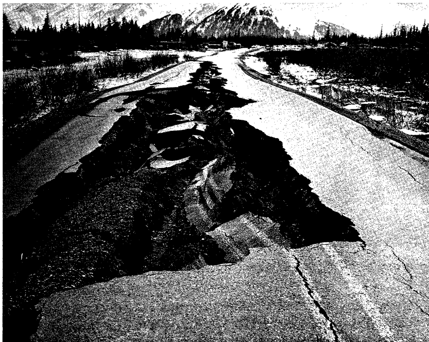
Earthquake cracks in Anchorage-Seward Highway near Portage, 1964.
