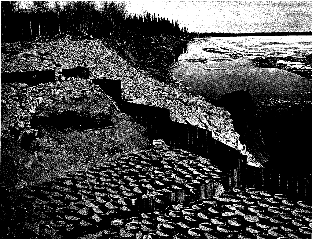
Gravel-filled drums behind sheet steel piling were one form of bank erosion control tried at Galena on the Yukon, 1964.
