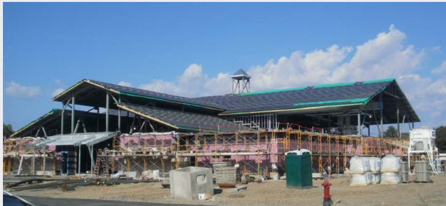
Construction work at the Armed Forces Reserve Center in White River Junction, Vermont.
