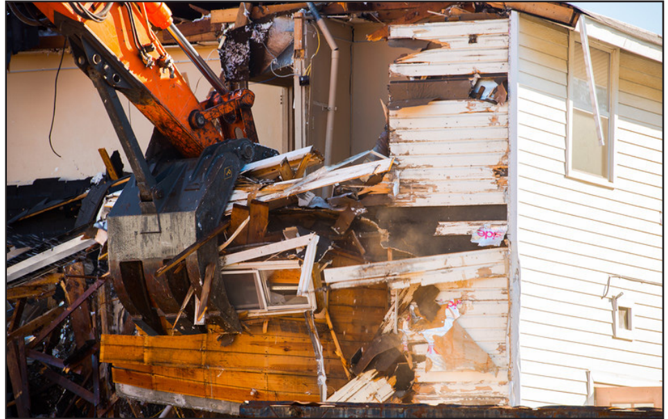
Demolition began Feb. 16 on Soldier's Plaza, Fort Benning, Georgia, to remove old World War II-era buildings and reduce the installation's footprint. (Photo by Patrick A. Albright)
