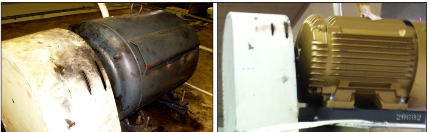
By downsizing the supply fan from a 40-horsepower one to a 30-horsepower one, a maintenance team at the Presidio of Monterey, California, saved replacement costs and long-term energy and usage costs. (U.S. Army Photo)
