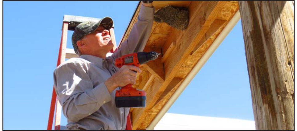
James Kulbeth, Directorate of Public Works Environmental Division biologist at Fort Carson, Colorado, installs five man-made mud nests onto the structure to encourage the cliff swallows to build their own nests. (U.S. Army Photo)
