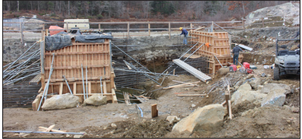
Renovation work at the Mine Lake Dam in West Point, New York, will help preserve the original historic structure while extending its life for another 100 years. (U.S. Army Photo)
