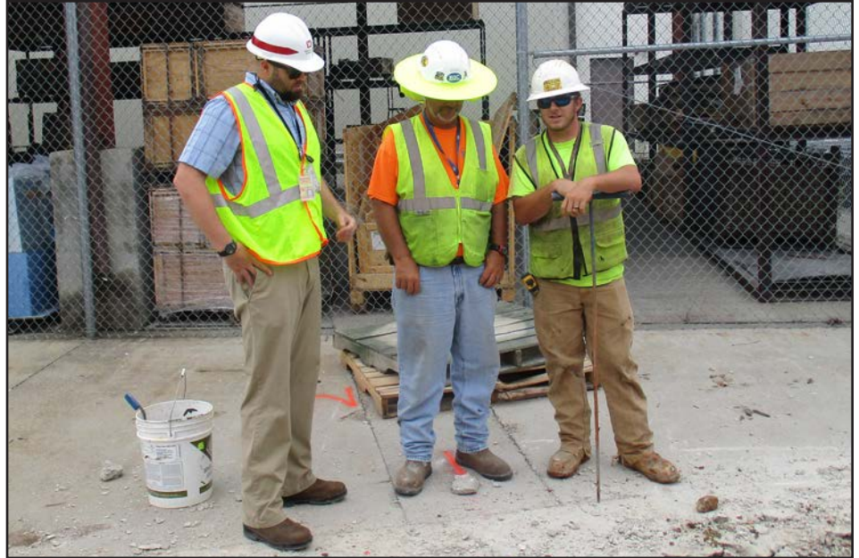
Chad McLeod, left, the area engineer at Anniston Army Depot, Alabama, reviews construction work with Keith Slick, center, project superintendent for Birmingham Industrial Construction, and Kevin Hightower, right, a pipe layer for Taylor Corp. (U.S. Army Photo)
