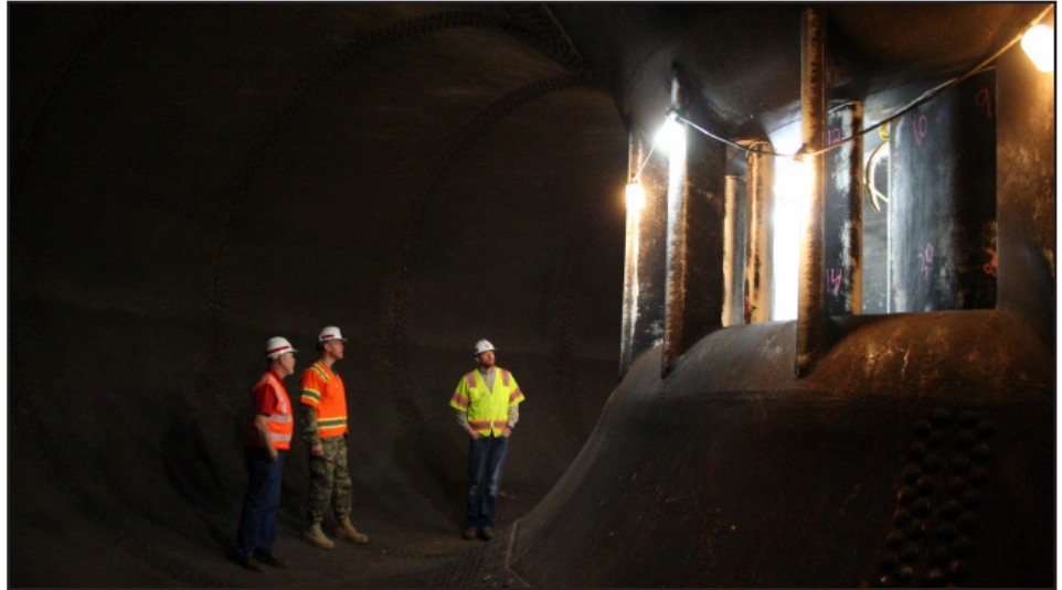
Fort Randall Operation's Project Manager Tom Curran, Omaha District Commander Col. John Henderson, and Fort Randall Power Plant Maintenance and Operations Manager Mike Schenkel inspect a dewatered hydropower unit's wicket gates from inside the scroll case. The unit has been set aside for cavitation repairs.
