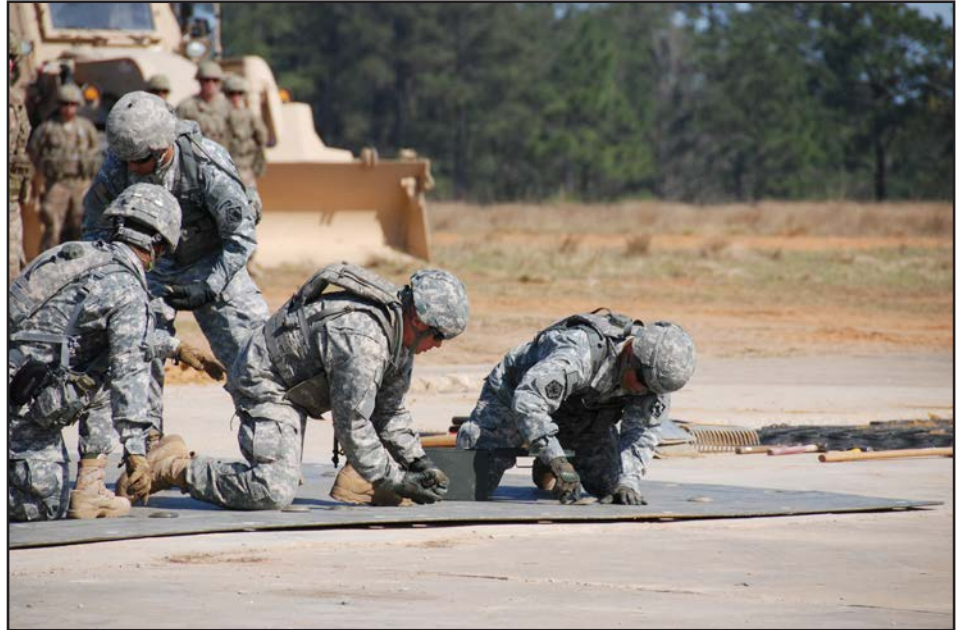
Soldiers from Fort Bragg, North Carolina, race to install fiber reinforced panels during an Airfield Damage Repair demonstration held March 17 at Fort Bragg. The U.S. Army Engineer Research and Development Center, the Maneuver Support Center of Excellence and Fort Bragg engineer units have been working on the project since January 2015. The intent is to upgrade the Army's airfield damage repair procedures, making them faster and more efficient. (U.S. Army Photo)
