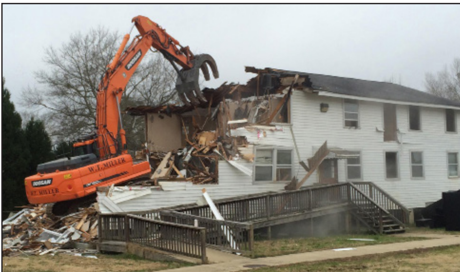
Soldiers Plaza building 2602, a World War II wood building used most recently as an administrative building, is demolished at Fort Benning, Georgia, under the Facilities Reduction Program, U.S. Army Engineering and Support Center, Huntsville. (U.S. Army Photo)
