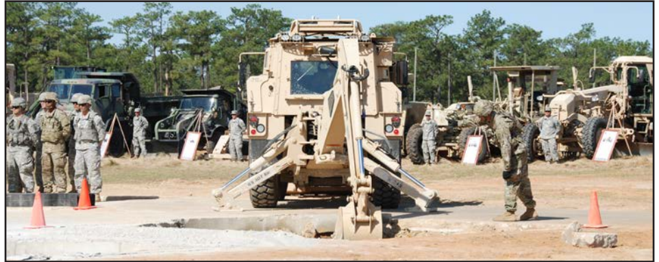
A Fort Bragg engineer guides the High Mobility Engineer Excavator through its paces at the Airfield Damage Repair Demonstration held March 17 at Sicily Drop Zone, Fort Bragg, North Carolina. U.S. Army Engineer Research and Development Center engineers and researchers collaborated on the demonstration with Soldiers as part of an Airfield Damage Repair upgrade project during the past year. (U.S. Army Photo)
