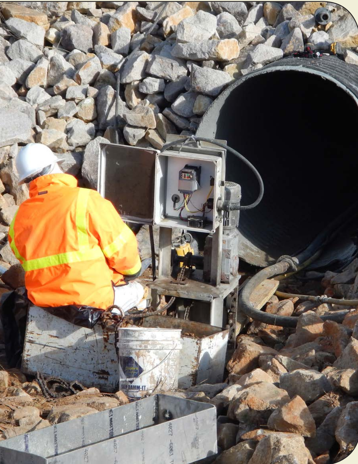
A technician controls application of geopolymer mortar liner to rehabilitate a steel storm drainage culvert at Simmons Army Airfield, North Carolina. (U.S. Army Photo)
