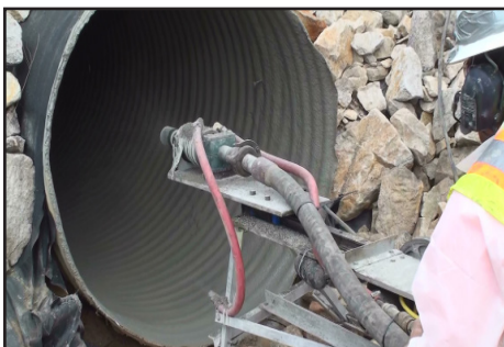
The spin-cast head is shown at the end of the first out of three passes. The unit has been pulled through the pipe while spraying the gray-colored geopolymer liner on the inside of the pipe. (U.S. Army Photo)
