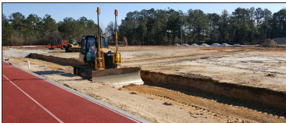
A contractor excavates the trench at Hercules Stadium at Pope Air Force Base in preparation for the artificial turf. (Photo by Leonard Booth)
