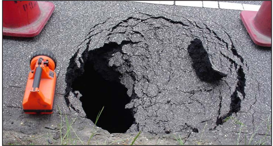
Poor drainage or compromised drain pipes under roads can lead to sink holes that undermine the road and cause serious issues, both for an installation and for a driver. (U.S. Army Photo)
