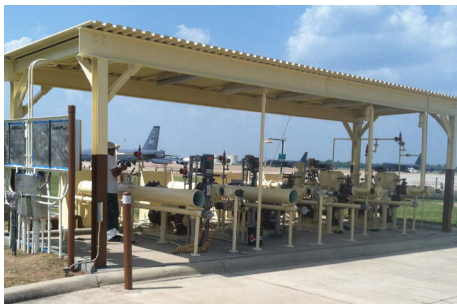
A recently renovated service control point ensures fuel is delivered
