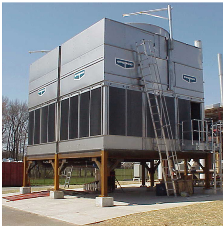
An energy savings performance contract at Aberdeen Proving Ground, Maryland, added a cooling tower to support two 750-ton chillers to operate 24x7x365 in a surety laboratory. (Presgraves)
