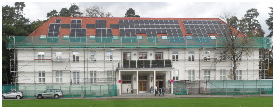
PV panels on the USAG Stuttgart installation
