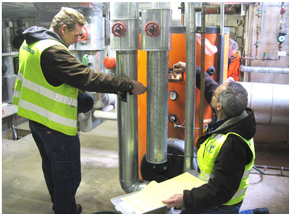
A project team inspects mechanical systems at Sembach Kaserne near Kaiserslautern, Germany, during an energy audit conducted for an energy master planning project aimed at achieving net-zero energy status by 2025. (USACE)
