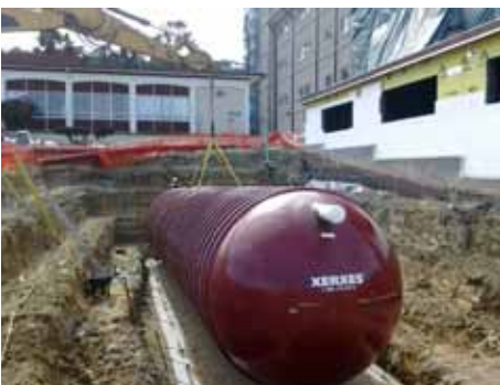
A 35,000-gallon tank is put into place next to a new general instruction building under construction at the Presidio of Monterey, Calif., March 25, 2013. (U.S. Army Photo by Jack Davies/Released)
