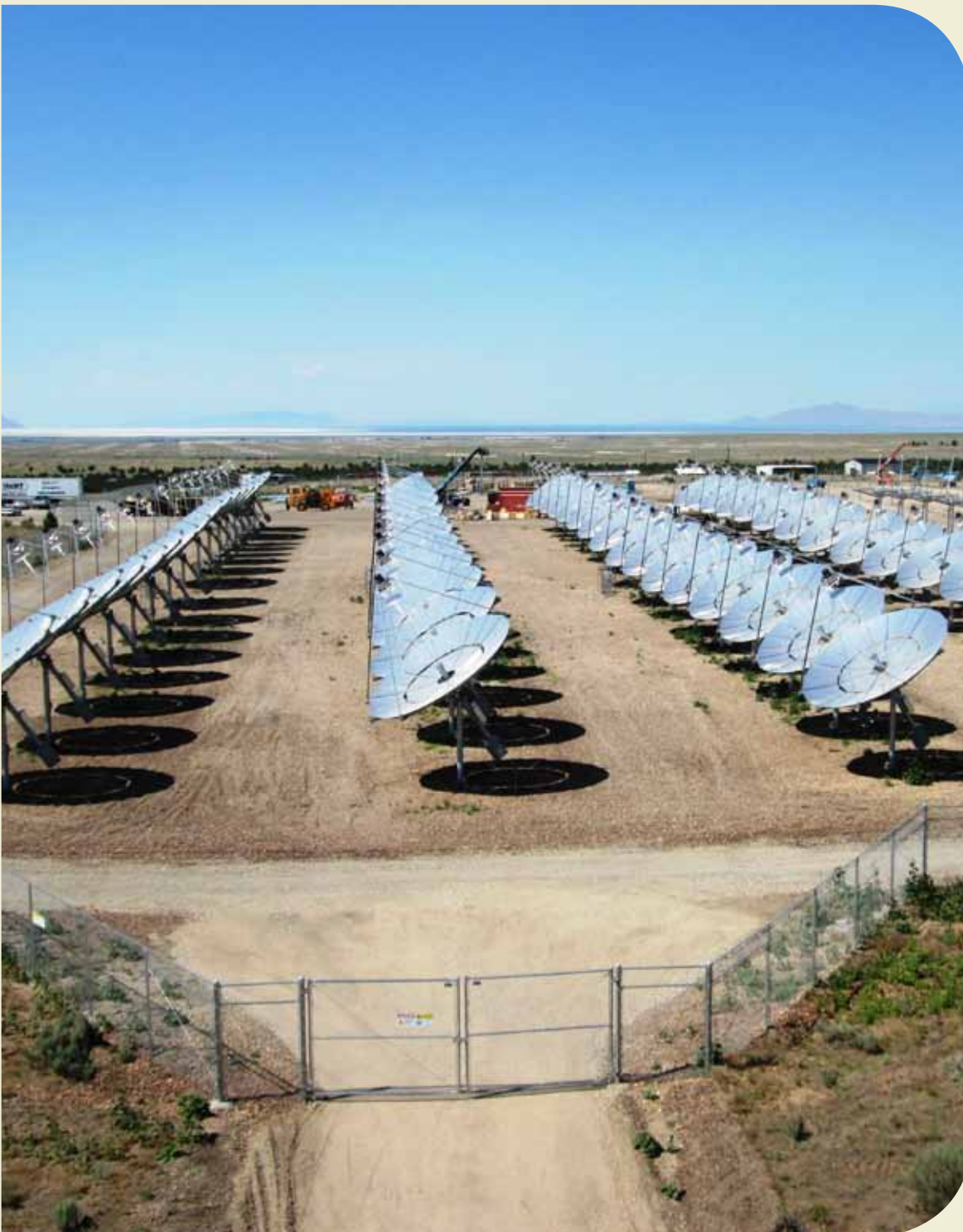
Stirling Solar Array at Tooele Army Depot will consist of 429 power units and is expected to provide 1.5 Megawatts of electricity. Complete article located on page 10.
