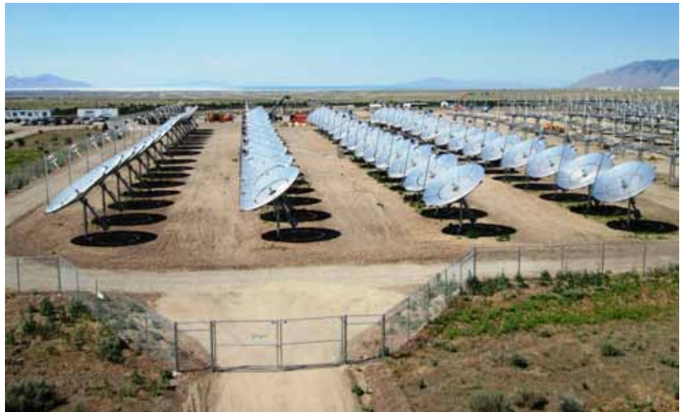
Stirling Solar Array at Tooele Army Depot, FY12 ECIP Project. This is the first block of 64 concentrating solar power units at Tooele Army Depot (TEAD). Upon construction completion, the solar array will consist of 429 power units and is expected to provide 1.5 Megawatts of electricity, which equates to approximately 30% of TEAD's total annual electric energy need. (Photo by Chris Beauchamp, Infinia Corp.)
