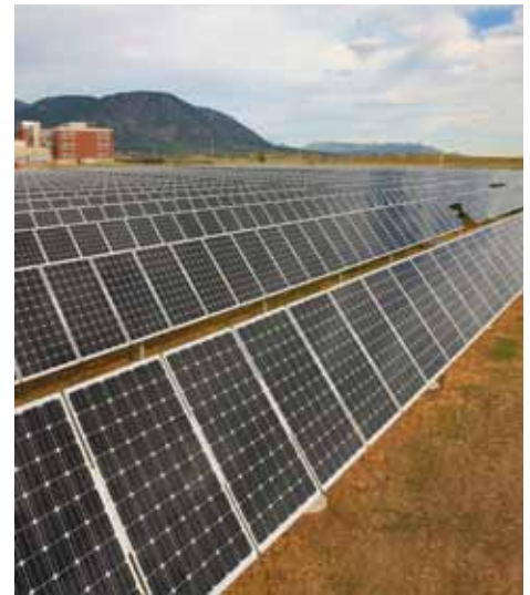
Fort Carson’s first U.S. Green Building Council platinum-level Leadership in Energy and Environmental Design certified facility, the 4th Armored Brigade Combat Team Brigade and Battalion Headquarters, features a 482 kilowatt ground-mounted, tracking photovoltaic system. (Photo by Harry Weddington, USACE)
