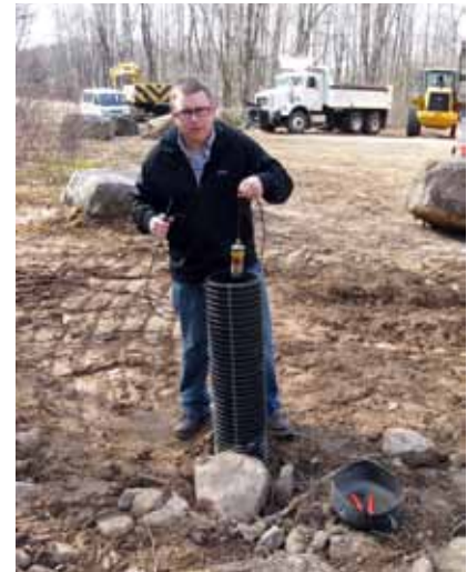
A Tobyhanna Army Depot employee uses leak detection technology as part of a regional water assessment. U.S. Army photo
