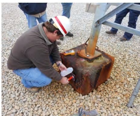
An ERDC engineer takes measurements on corrosion-damaged power transmission towers at Sam Rayburn Dam near Jasper, Texas. Photo by U.S. Army Corps of Engineers
