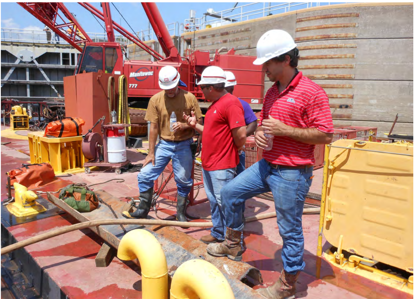
ERDC researchers work with Tulsa District field engineers at Newt Graham Lock and Dam during maintenance and repair operations. Photo by U.S. Army Corps of Engineers
