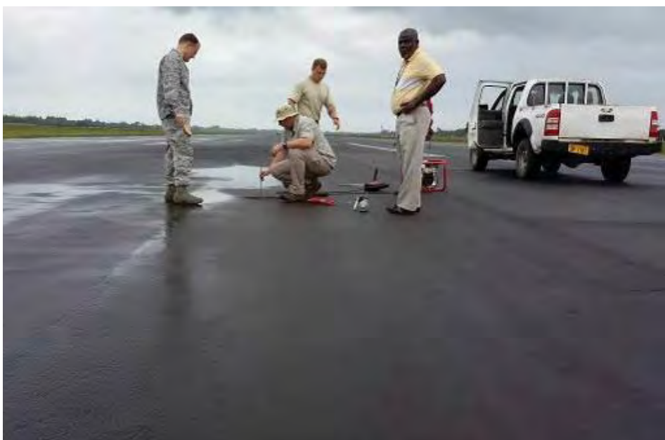
A depression, the result of a failed subgrade and the source of multiple issues, is examined at Roberts International Airport, Monrovia, Liberia. Photo by U.S. Air Force
