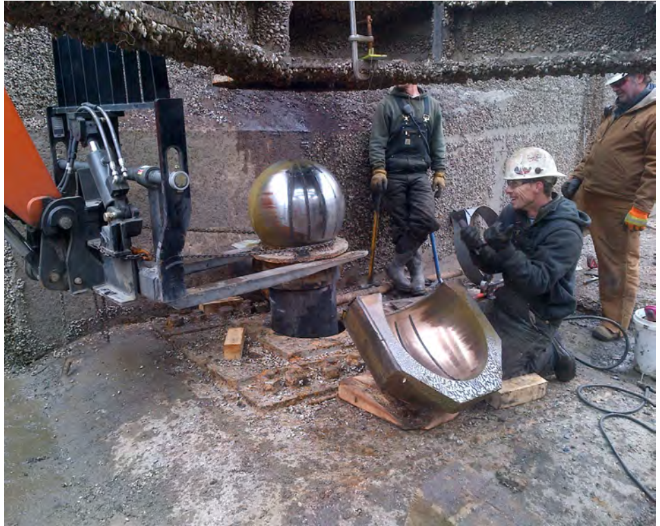
Illinois Waterway Maintenance Crew members, Craig Williams, Cory Bowen and Mark Hanson remove the pintle ball and bushing from the lower right sector gate at the T.J. O'Brien Lock. Photo by Brady Beckman
