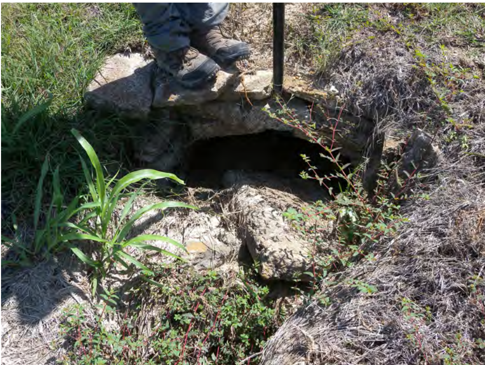
Inventory and Aging Infrastructure. Survey grade information of stormwater infrastructure was taken. Examples of aging stormwater systems was evident and recorded during the inventory.
