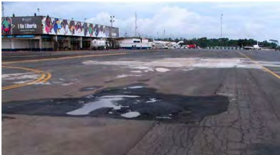
With pavement that is roughly 40 years old, Liberia's Roberts International Airport struggled under the demand for humanitarian aid in the midst of the Ebola Virus crisis. Photo by U.S. Air Force
