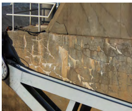
A severe alkali-silica reaction is shown in a dam pier at David Terry Lock and Dam in Pine Bluff, Arkansas. Photo by U.S. Army Corps of Engineers
