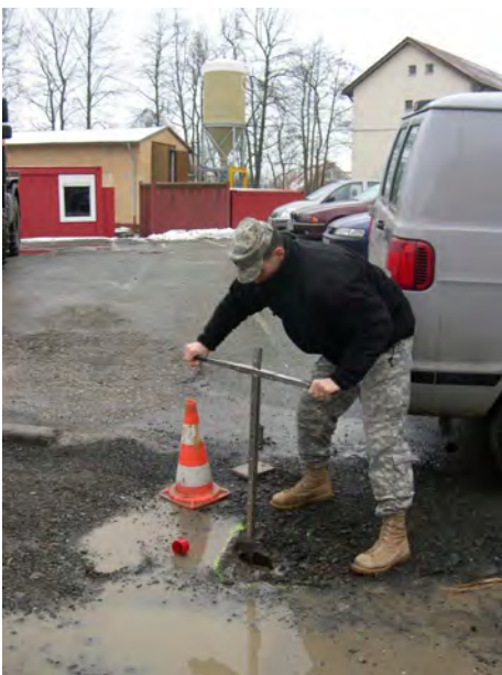
An Army lieutenant checks valve operation on a 12” line at an installation. Courtesy photo
