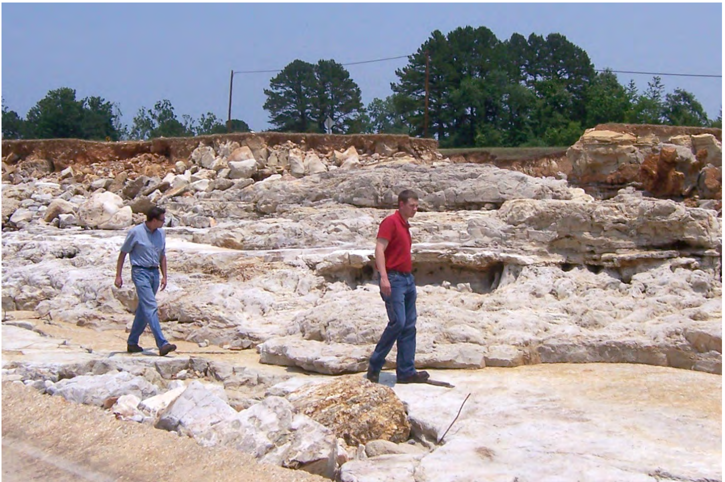
Gary Lee, chief, Design Branch, left, and Kyle Arentsen, structural engineer, inspect the Wappapello Lake, Missouri, spillway failure during the Great Flood of 2011. Courtesy photo
