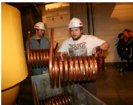
Electrician Connor Florey (left) assists mechanic Bryce Stasch (right) with new cooling coils to be installed on the hydropower units at Fort Randall Dam. Photo by Al Barrus
