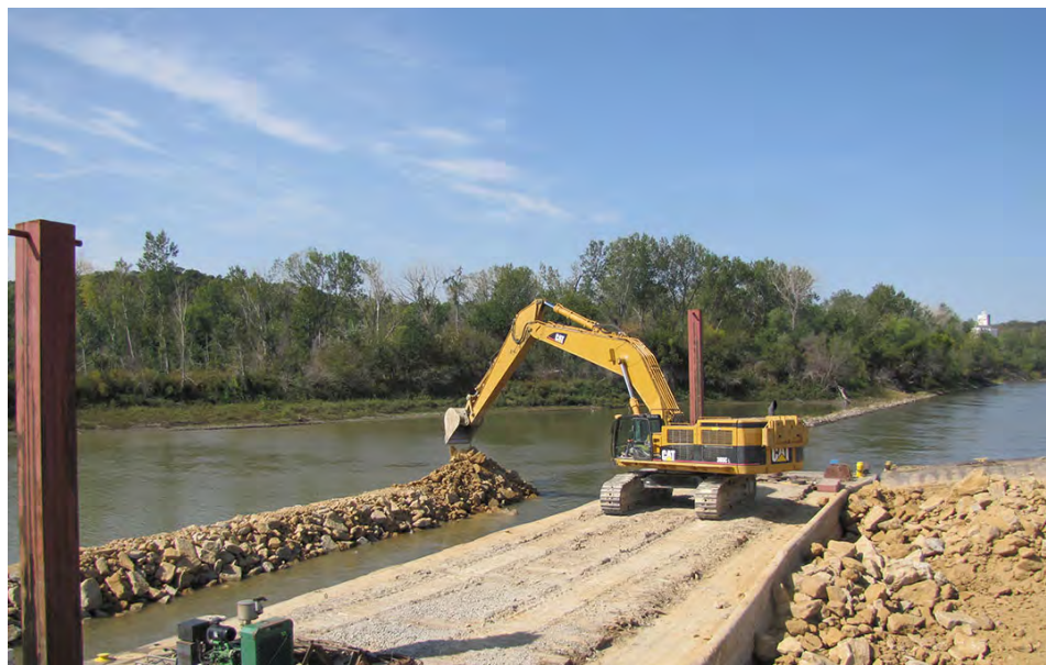
Contractor placing rock on a Missouri River revetment. Photo by Dereck Wansing
