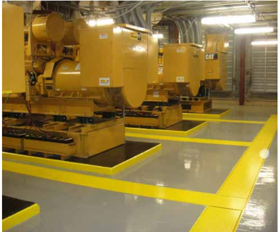
Other OMEE examples include mechanical room industrial boilers and generators.
