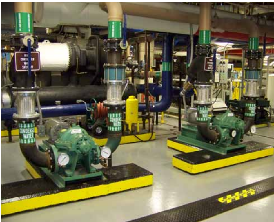
This is an example of pumps found in a mechanical room in a hospital. The OMEE program maintains the facility and performs preventative maintenance and repairs to these type systems.
