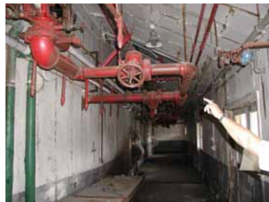
PCBs have been found in paint such as this red coating on pipes in a military industrial complex. Photo courtesy of ERDC-CERL
