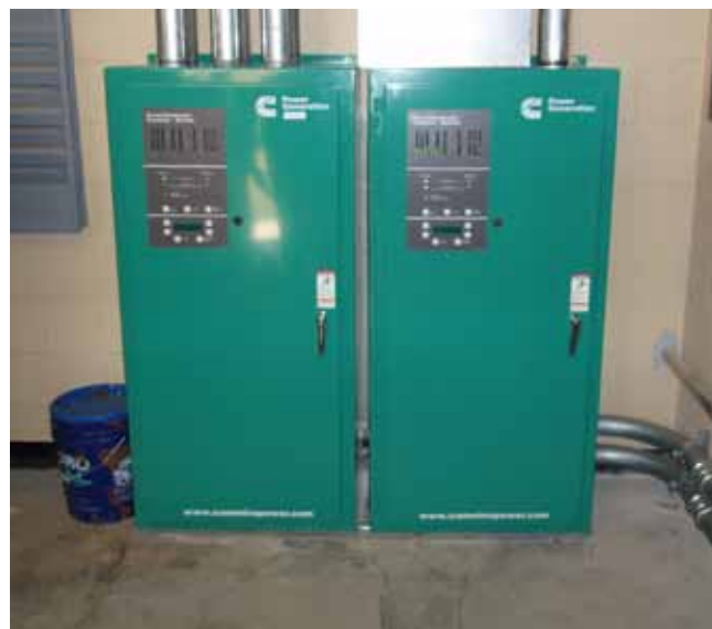
Automatic Transfer Switch (ATS)
