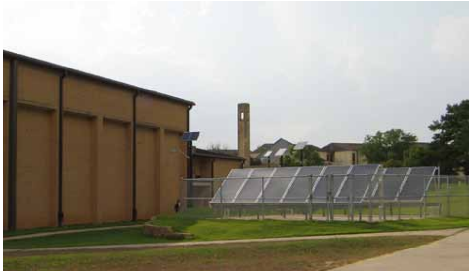
Solar panels at Fort Polk
