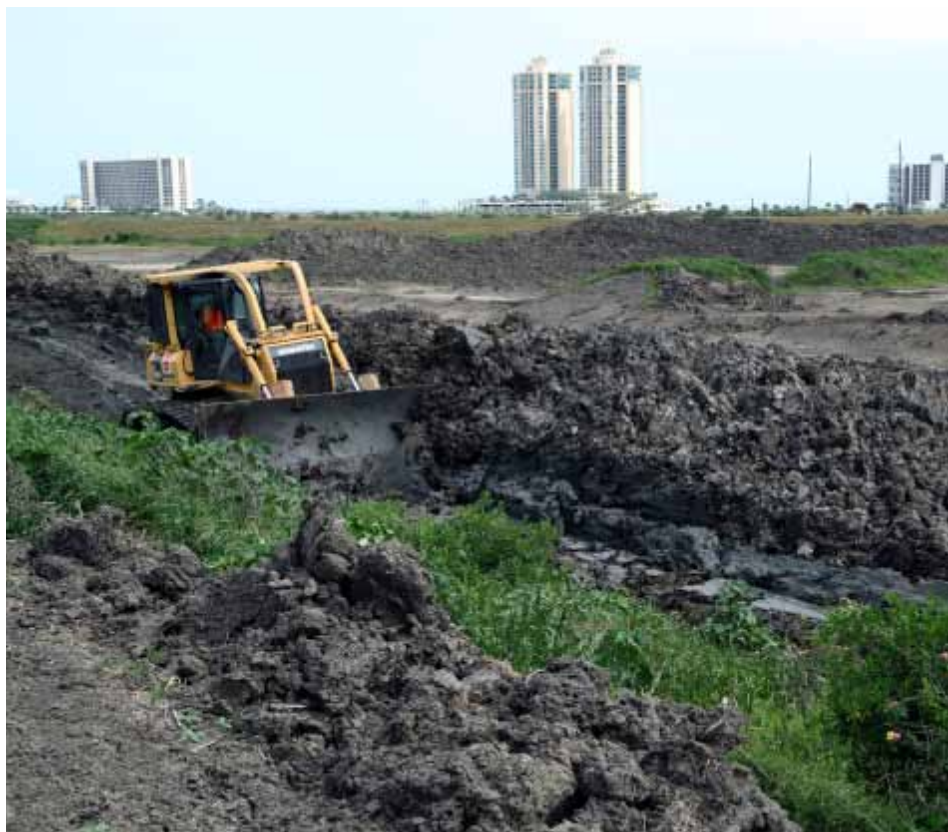
Heavy equipment operators construct dewatering ditches at the San Jacinto Placement Area as part of $1,382,700 contract to provide outflow of excess water to increase the placement area's capacity to hold more dredge material.
