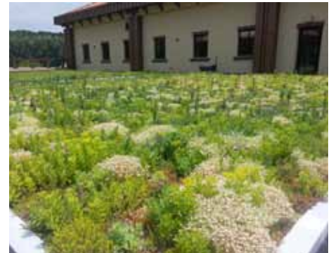
The U.S. Army Corps of Engineers Far East District installed a roof-top garden on the new health and dental clinic at Camp Carroll at U.S. Army Garrison Daegu, Republic of Korea, making it the first green roof on a U.S. military facility in the country.
