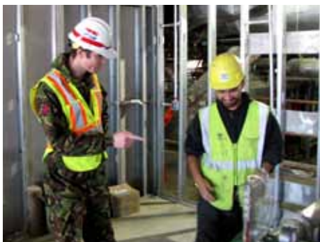
Capt. Ben Hancock works with a Fort Detrick contractor to test ducts at the USAMRIID project to ensure containment and that all specifications are met as part of the quality assurance process. Photo by Brittany Bangert
