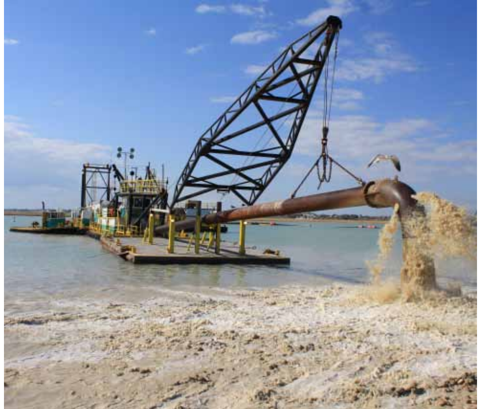
1st photo - The spill barge "Shamrock" places material to construct an underwater levee that is part of a Beneficial Use Site to provide a shallow water sea grass habitat along the south side of the new channel. Photo by Kenneth (Chip) Worley.
