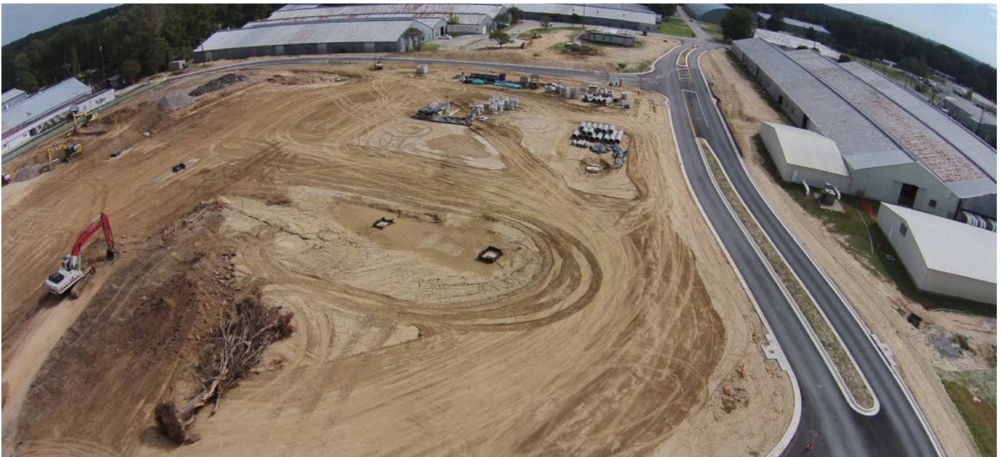
Aerial photograph of the construction site for the new headquarters building at the U.S. Army Engineer Research and Development Center in Vicksburg, Mississippi. Construction of the 142,000 square foot building with a four-story southern wing and a three-story northern wing is set for completion in 2017.
