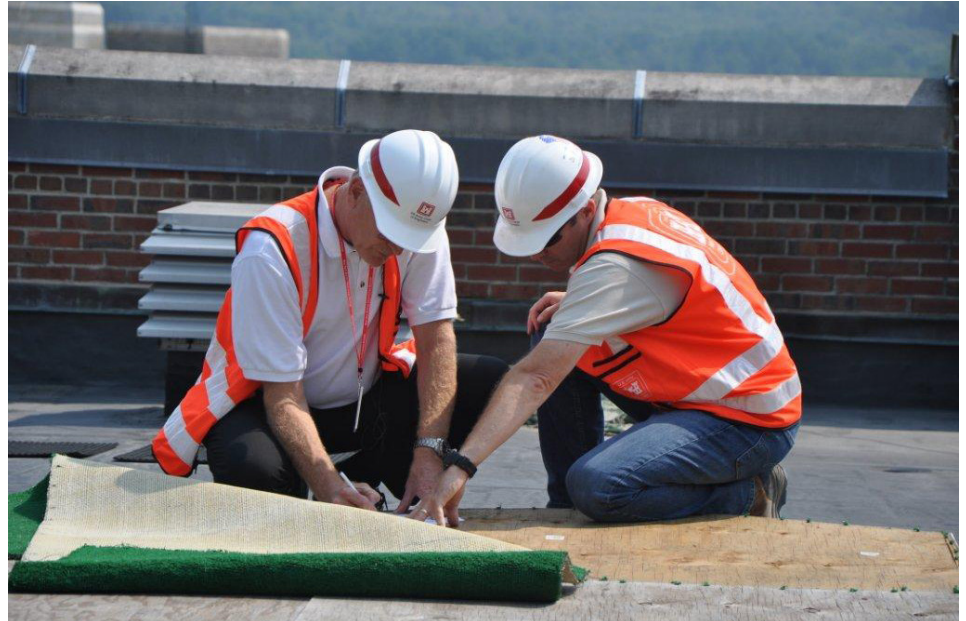
U.S. Army Corps of Engineers personnel work on the Davis Barracks construction site at West Point, New York. (Photo by James D'Ambrosio)
