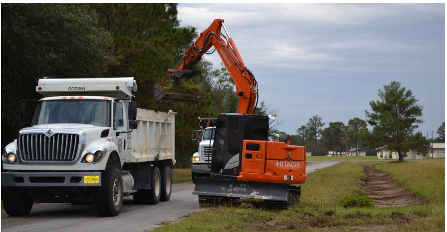
Excavation equipment removes soil for the Camp Blanding swale cleaning project. (U.S. Army Photo)
