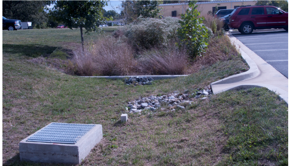
Bioretention with forebay and overflow inlet in parking lot at Fort Meade, Maryland. (U.S. Army Photo)
