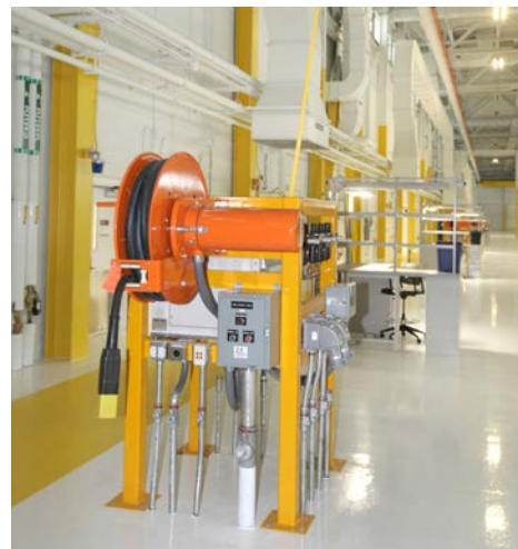
The 10-ton cranes in the 404th Aviation Support Battalion's Net Zero hangar at Fort Carson, Colorado, support the maintenance of the 4th Combat Aviation Brigade's 113 helicopters, which include CH-47 Chinooks, UH-60 Blackhawks, OH-58 Kiowas and AH-64 Apaches. (Photo by Harry Weddington)
