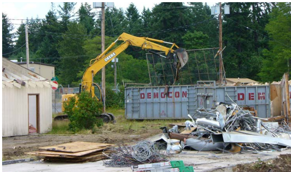
An excavator separates debris material from salvageable material at Joint Base Lewis McChord, Washington, as the installation works to meet waste diversion requirements. (Photo by Thomas Napier)
