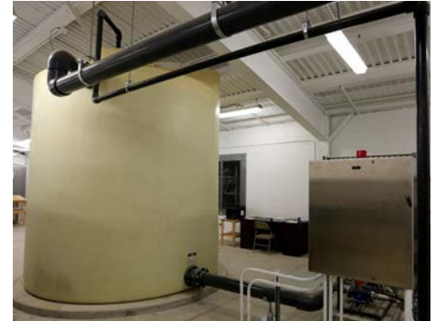
Tobyhanna Army Depot completed installation of its reclaimed water system as part of the upgrades of the Waste Water Treatment Plant. In fiscal year 2015, it resulted in a 90 percent reduction from the average monthly potable water use at the plant, with a savings of $50,497. (U.S. Army Photo)
