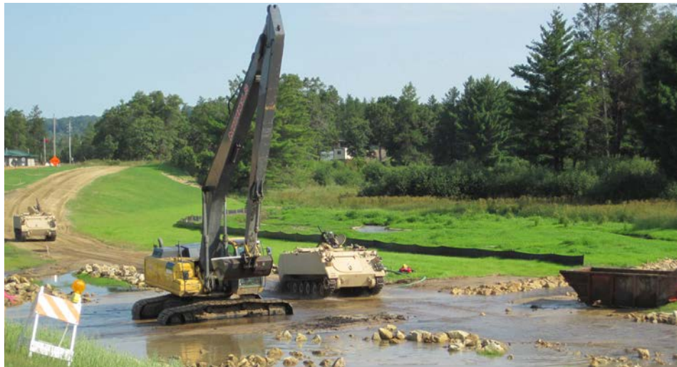
Army M113 Armored Personnel Carriers move through the newly constructed La Crosse River low water crossing designed to support heavy tactical vehicles. (U.S. Army Photo)
