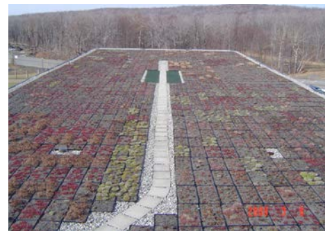
Green roof retrofit on industrial building at Tobyhanna Army Depot, Pennsylvania. (U.S. Army Photo)
