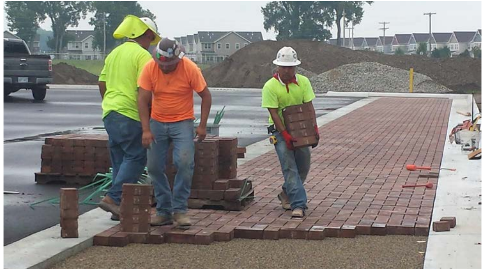
Workers install "smart" permeable pavers at a parking lot at Seitz Elementary School. (Photo by Chris Otto)
