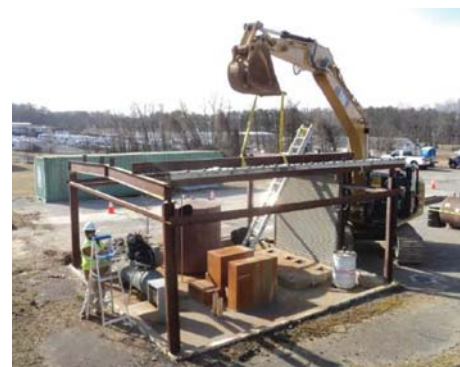
The groundwater collection and treatment system at OU-2 was deconstructed after the site reached regulatory closure. System deconstruction, as opposed to demolition, maximized the amount of material suitable for recycling. Of the total 90.2 tons of material associated with the treatment system, 7.17 tons of steel and 82.59 tons of aggregate were recycled (recycling rate of 99% material by weight).
