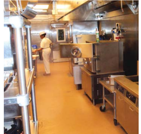
Large kitchen hoods like this one in a dining facility at Fort Carson, Colo., are candidates for variable flow exhaust controls. (ERDC)
