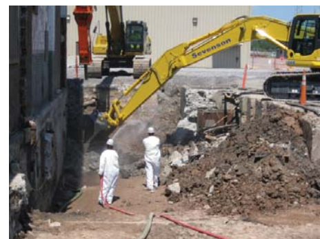
Excavation in progress at the Linde FUSRAP site showing subsurface remediation adjacent to an existing building
