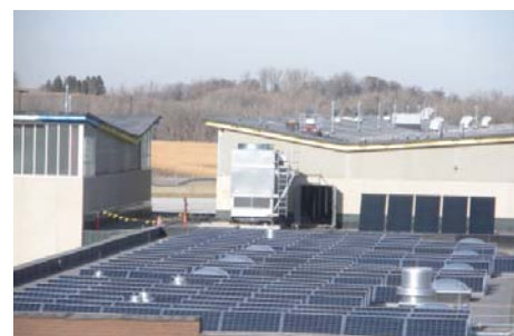
A 40kW solar photovoltaic system on the new Field Maintenance Shop at the Arden Hills Army Training Site. The system will satisfy about 6.5% of energy requirements of the building. This is the first use of solar energy for the Minnesota Army National Guard and more is planned.
