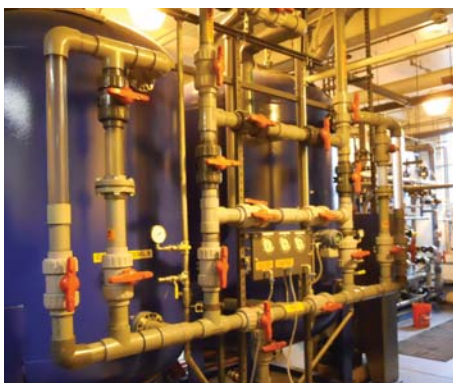
Process tanks at the Canal Creek Groundwater Treatment Plant at Aberdeen Proving Ground
