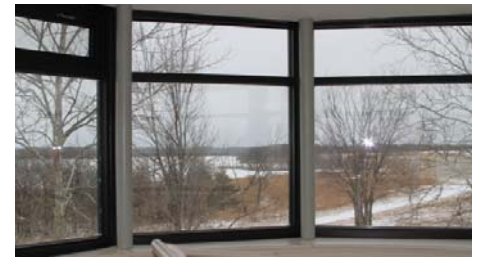
The drafty, 30-year-old second story window at the Smithville Lake Visitor Center was replaced, causing employees to notice an immediate difference. (Amy L. Phillips)
