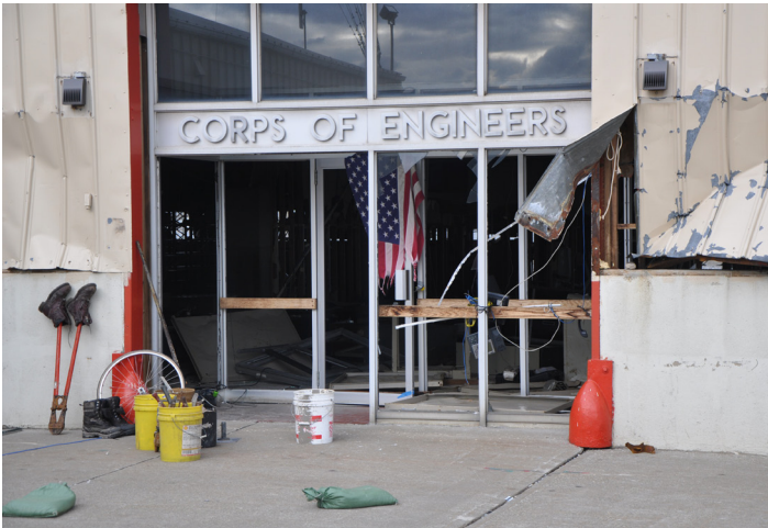
New York District's Caven Point Marine Terminal in Jersey City, N.J., was devastated by Hurricane Sandy's powerful storm surge as seen in this Nov. 2, 2012, photo of the facility's main entrance after the storm. (photo by Chris Gardner, New York District)
