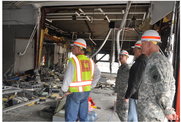
U.S. Army Corps of Engineers Deputy Commanding General Maj. Gen. Ken Cox surveys the severe damage at Caven Point on Nov. 2, 2012, with New York District leaders after Hurricane Sandy's storm surge devastated the facility. (photo by Chris Gardner, New York District)
