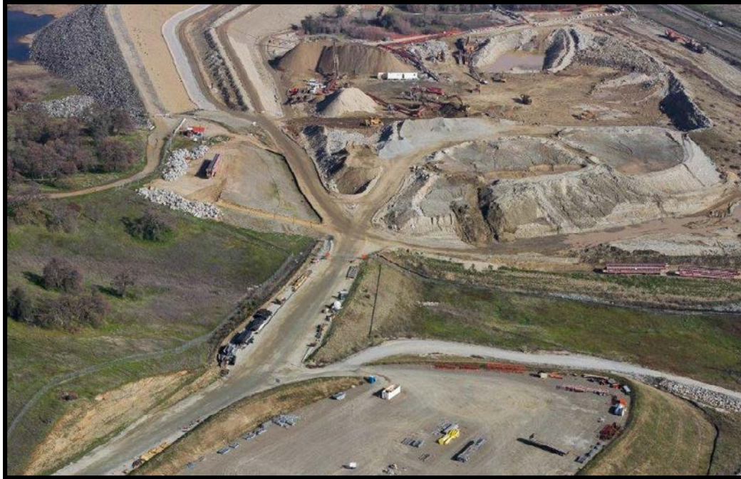
Photo 7. MIAD East Area and adjacent lands. View from the west looking east. MIAD East Area is in upper portion of photo, while some of the MIAD West Area is in lower portion.
