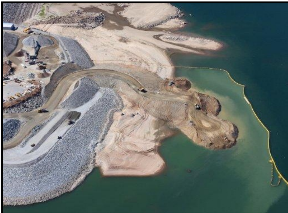
Photo 8. Overlook In-Lake Disposal (OILD) site and adjacent areas. View from the east looking west. Rip-rap area in lower left is a portion of the spur dike. Soil and equipment projecting into the lake from the spur dike are within the OILD site.
