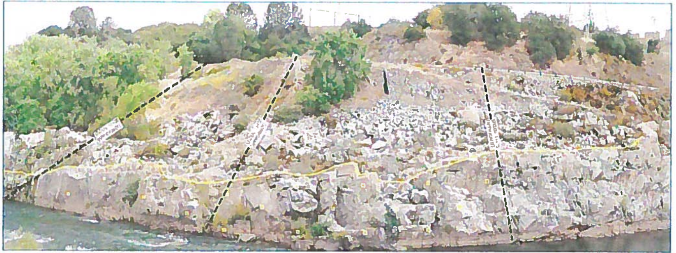
Figure 1. Approximate rock bolt locations on the right bank of the American River
