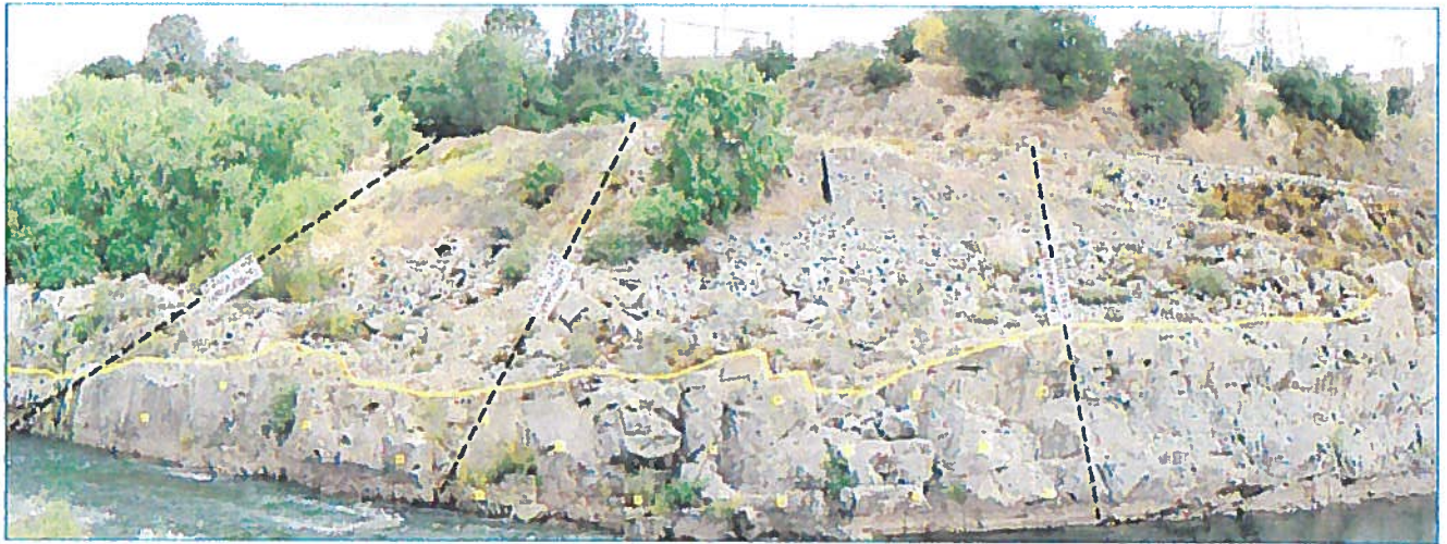
Figure 1. Approximate rock bolt locations on the right bank of the American River
