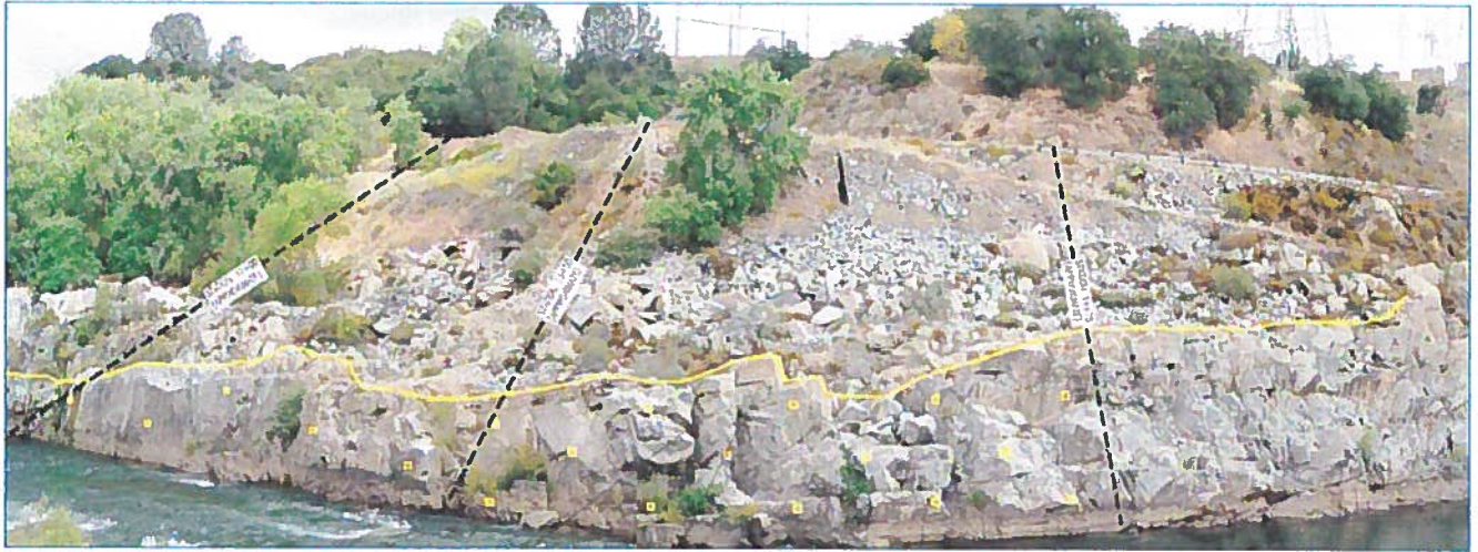
Figure 1. Approximate rock bolt locations on the right bank of the American River
