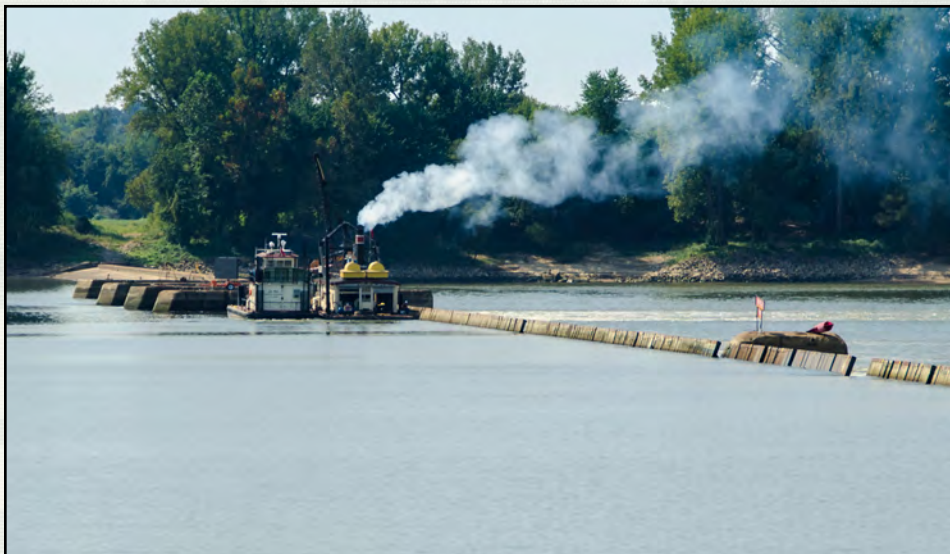
The workboat raises wickets on Dam 52. At right the three-wicket gap in the dam is visible.
