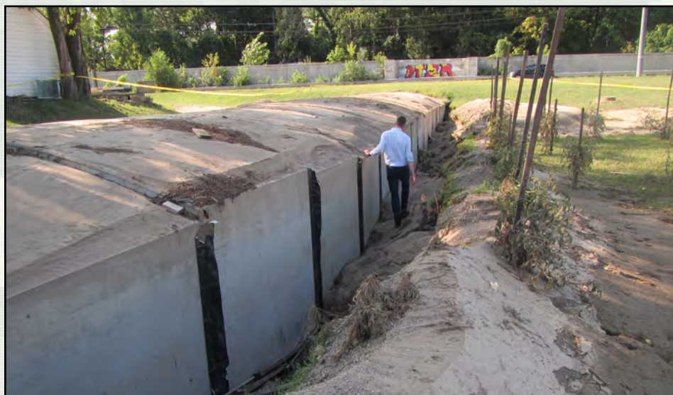
Pictured is a segment of the precast concrete arch culvert the Corps constructed as part of the flood risk management project in Cincinnati. The joints between the sections have separated and the alignment has shifted. Erosion is also present at right.
