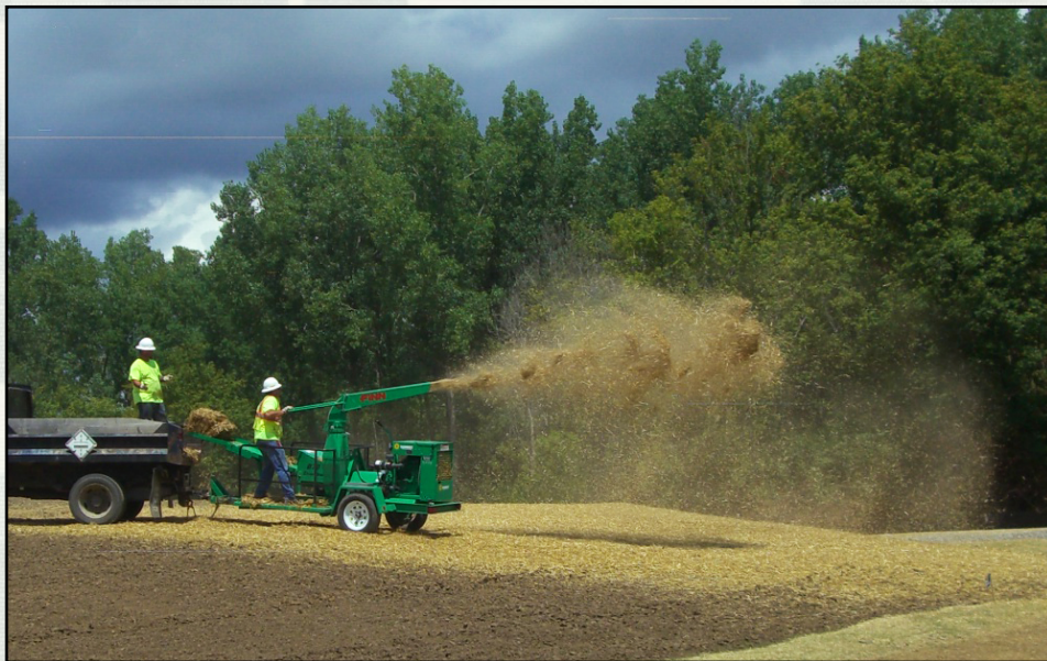
Contractors seed the soil cover at the former Lockbourne landfill, Columbus, Ohio, in August.
