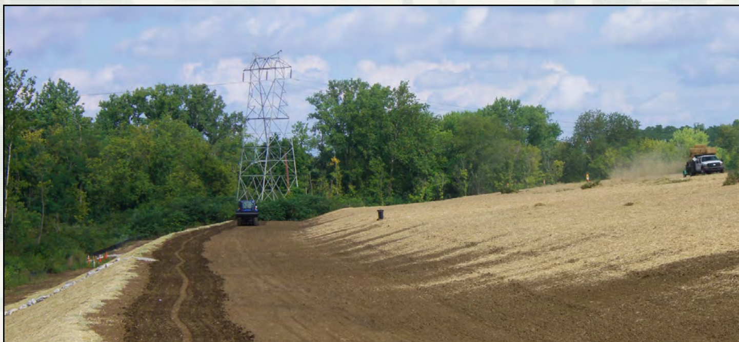
The 23-acre Lockbourne landfill cap is now complete, comprised of 24 inches of compacted soil and six inches of topsoil to create a barrier to prevent exposure to any contaminants.
