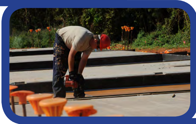
U.S. Air Force personnel perform construction at the Northwest Field site on Andersen Air Force Base, Guam, January 2009.
