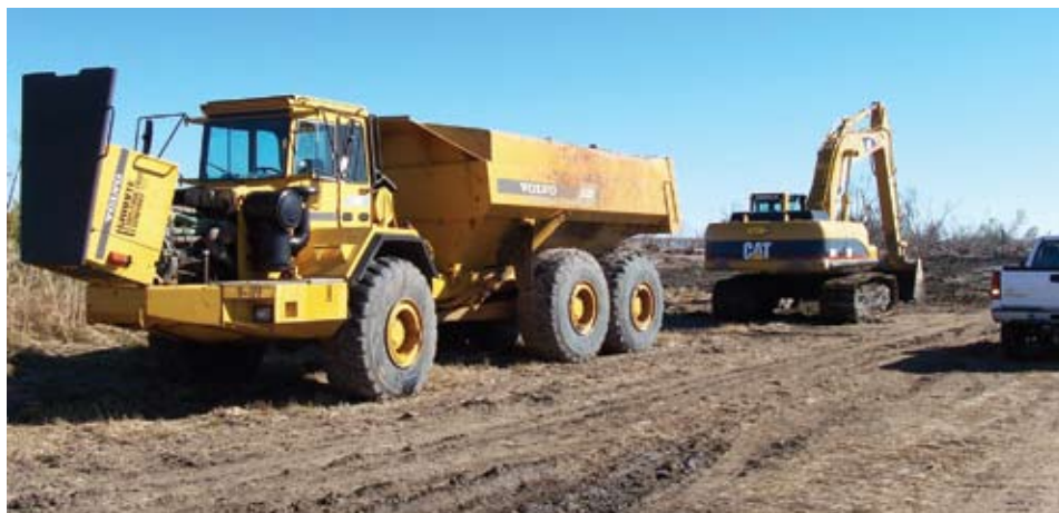
Top and Bottom Photos: Levee reconstruction post Hurricane Katrina. St. Bernard Parish, LA. August 2005
