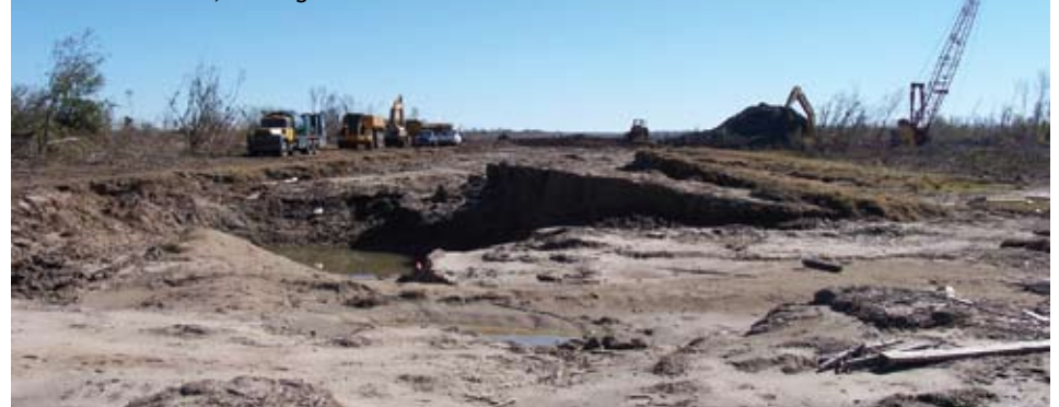
Levee damaged due to overtopping. Hurricane Katrina. St. Bernard Parish, LA. August 2005
