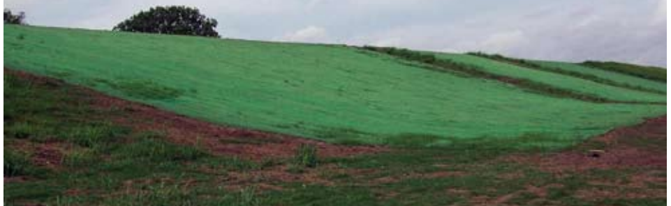
Repaired and replanted levee. Dallas, TX— Courtesy of City of Dallas Flood Control District
