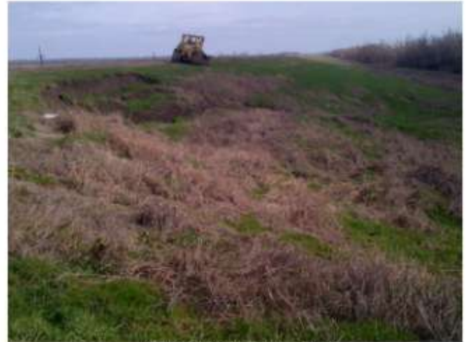
(Typical MRL Levee Slide)
