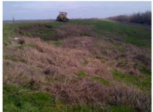
(Typical MRL Levee Slide)
