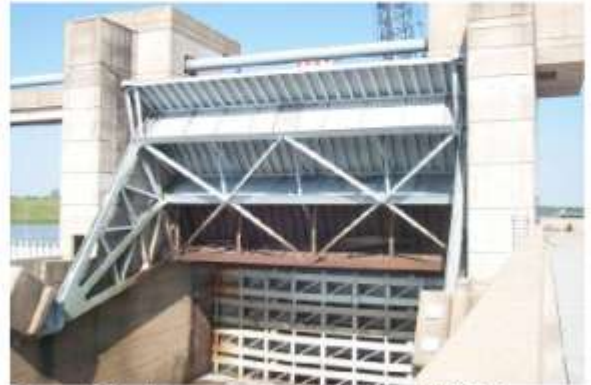
Figure 1. Previous repairs to Tainter Gates at L&D #1 (Boggs)
