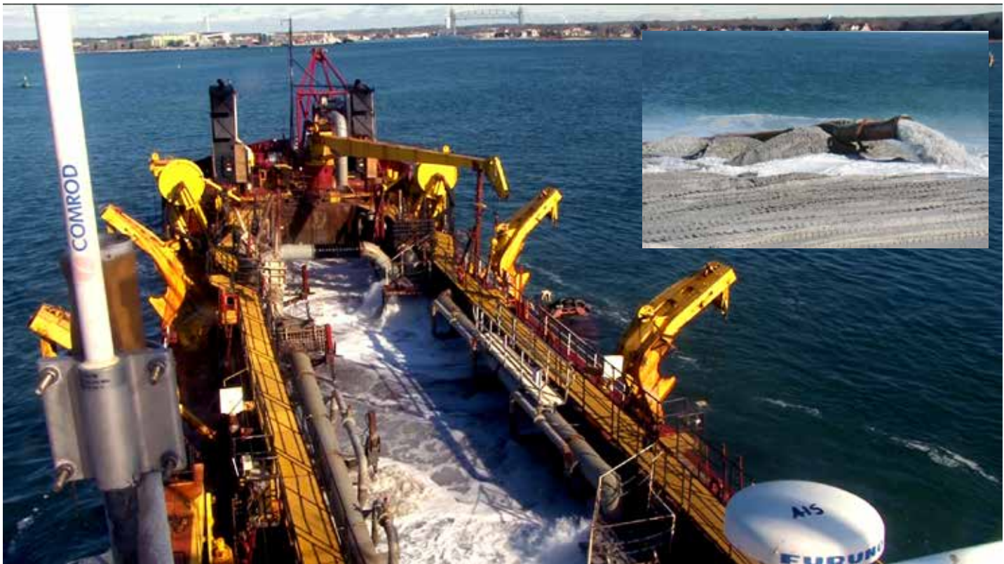
The hydraulic dredge operating in the canal. (inset) Sand being pumped onto Town Neck Beach.
