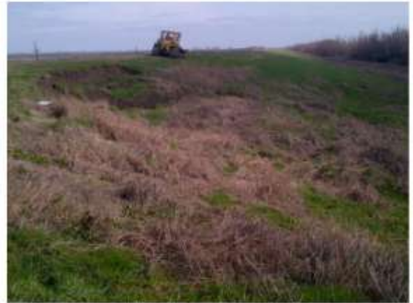
(Typical MRL Levee Slide)
