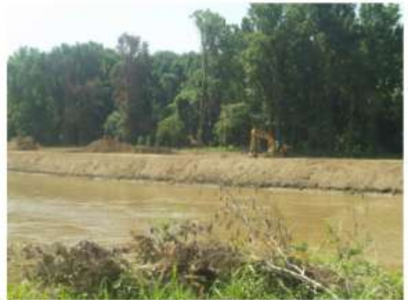
Construction along the bank of the Tallahatchie River Item 6B near Phillip, MS.
