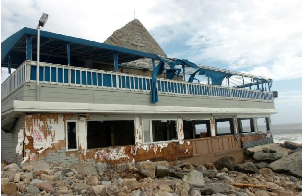
Figure 4. Damage to Historic Coast Guard House Restaurant
