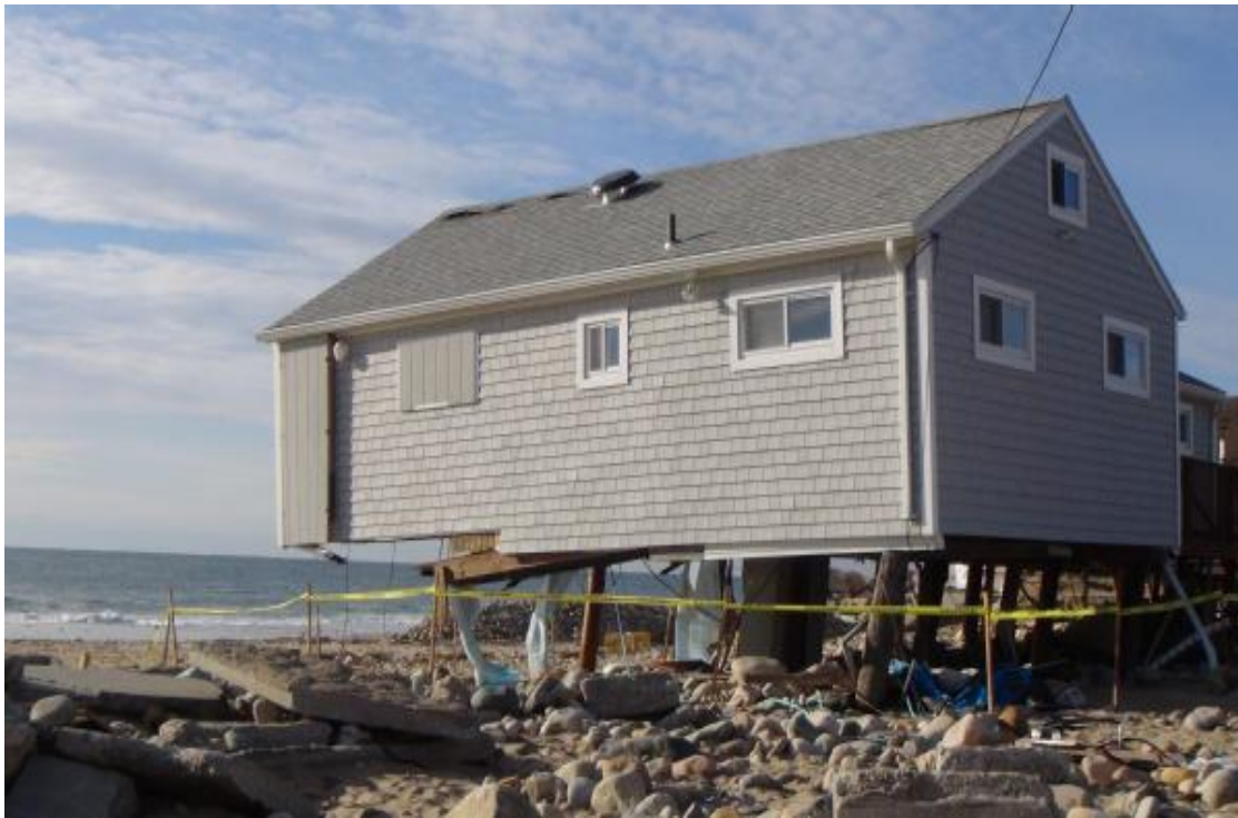
Figure 9. Westerly, Rhode Island home facing Misquamicut Beach damaged following Hurricane Sandy (FEMA Photo)
