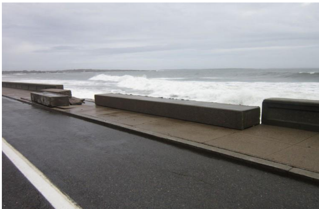
Figure 3. Portion of the Narragansett Seawall overturned during Sandy
