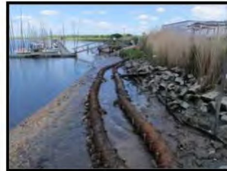
BEFORE: Day of installation of coconut-fiber (coir) logs and mats in New Jersey's Heislerville Fish and Wildlife Management Area in May of 2010.
