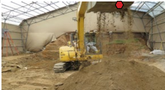
Above: Engineering Control Structure, tan tent, and other aspects of the multi-layered approach to public safety at the 4825 Glenbrook Road cleanup site are visible among the homes in the Spring Valley neighborhood in the District of Columbia, Feb. 4, 2016. (Courtesy photo)
