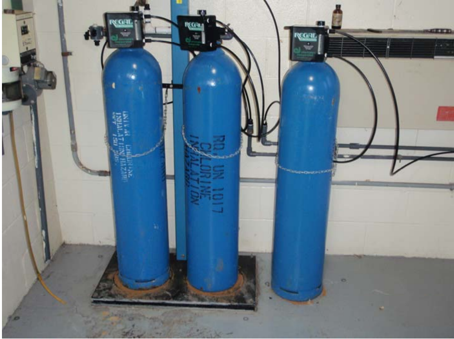
Chlorine Gas Tanks for Water Disinfectant Treatment
