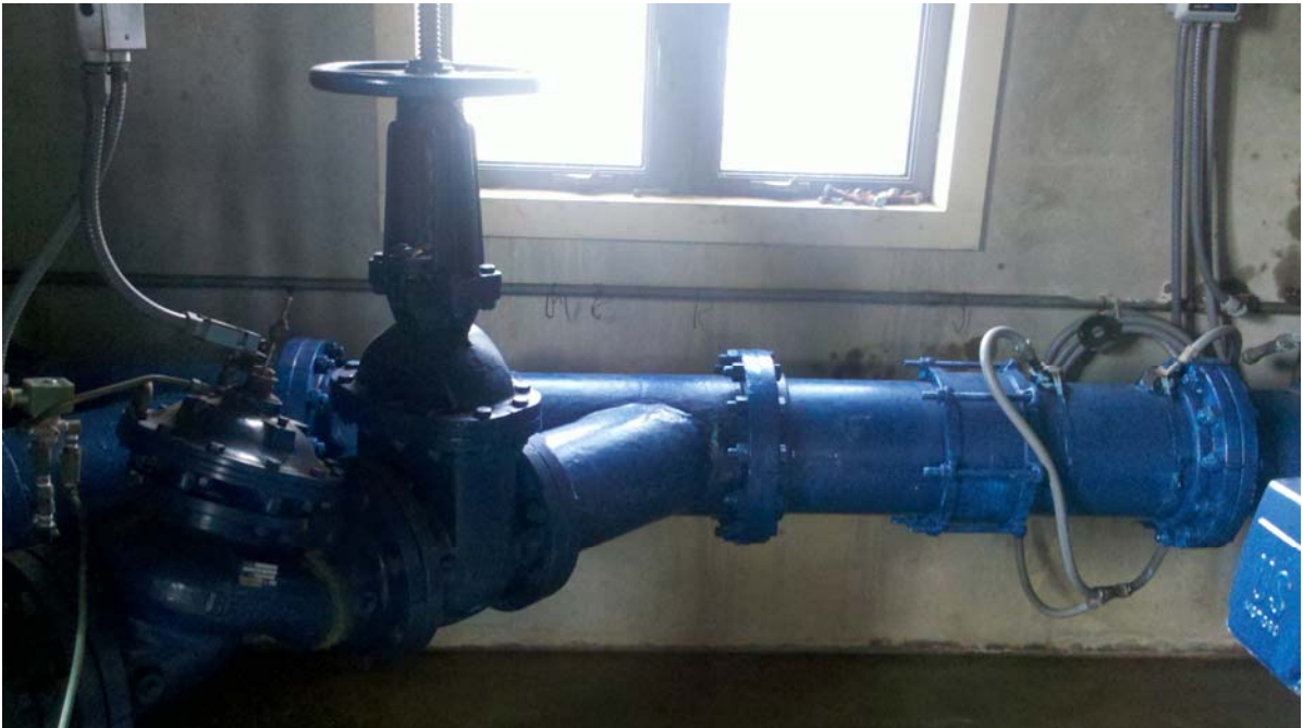
Plant Effluent Flow Meter in Pipe Gallery
