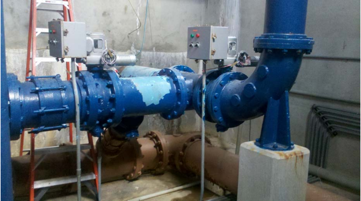
Electric Actuators in Pipe Gallery
