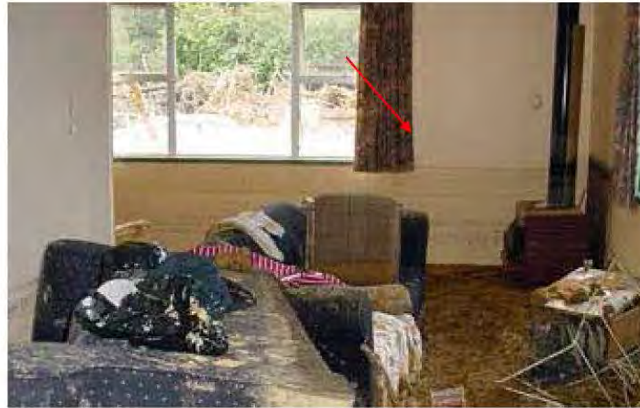
Figure G - 2. Example picture of a mud line on the inside of a building.
