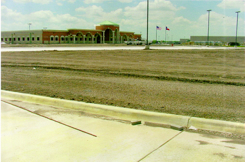
New county jail facility (taken while still under construction) west of and adjacent to the proposed BPS site.
