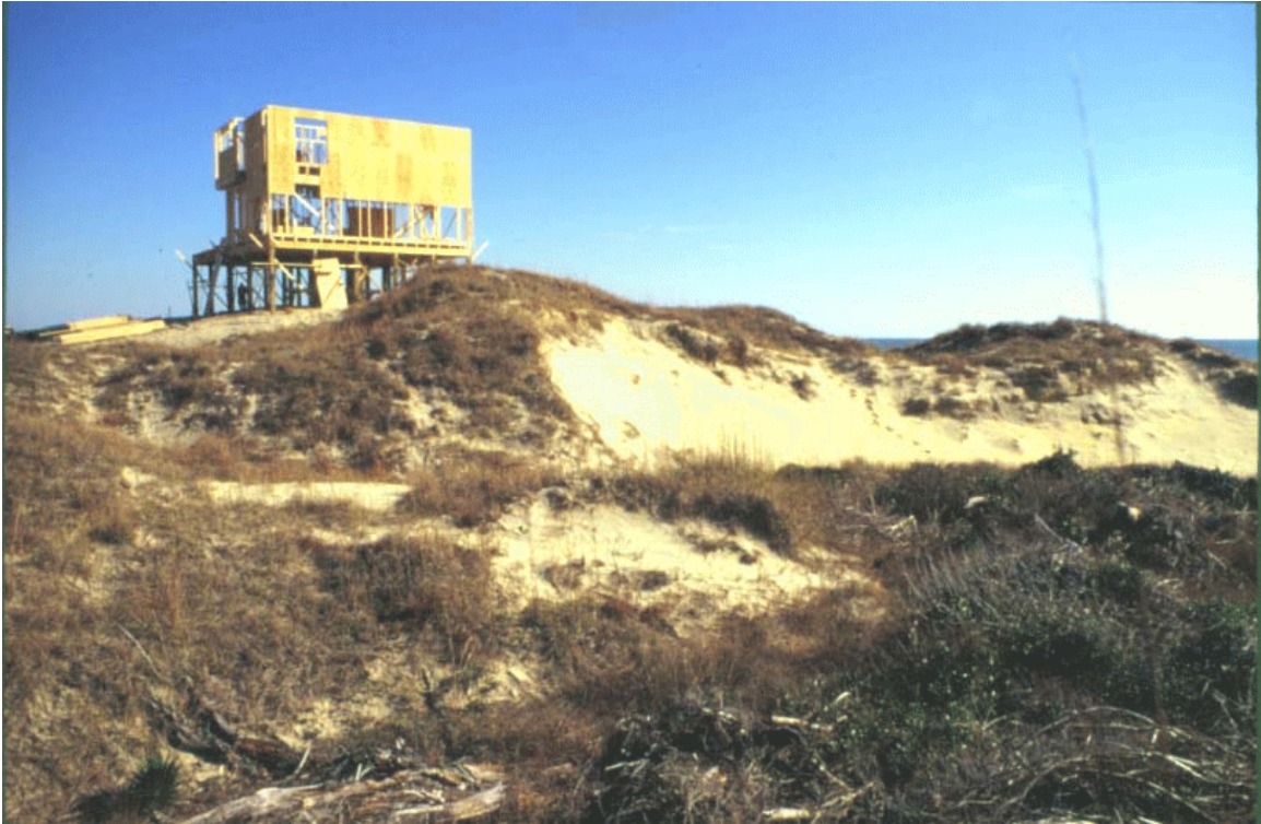
Figure 5: House under construction with piling 16 feet below grade (Class 1c) on high-elevation dune (Type A). Dune elevation above +16 feet NGVD makes erosion failure more likely. Location: Emerald Isle NC.
