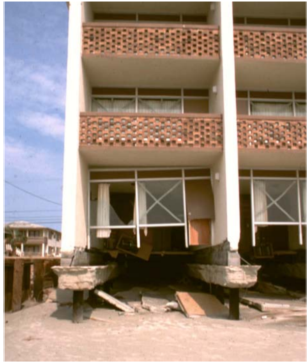
Figure 9: Piling-supported hotel after failure of unsupported, first-floor slab (Class 2b) on low-elevation shoreline (Type B). Location: Horry County after Hurricane Hugo.
