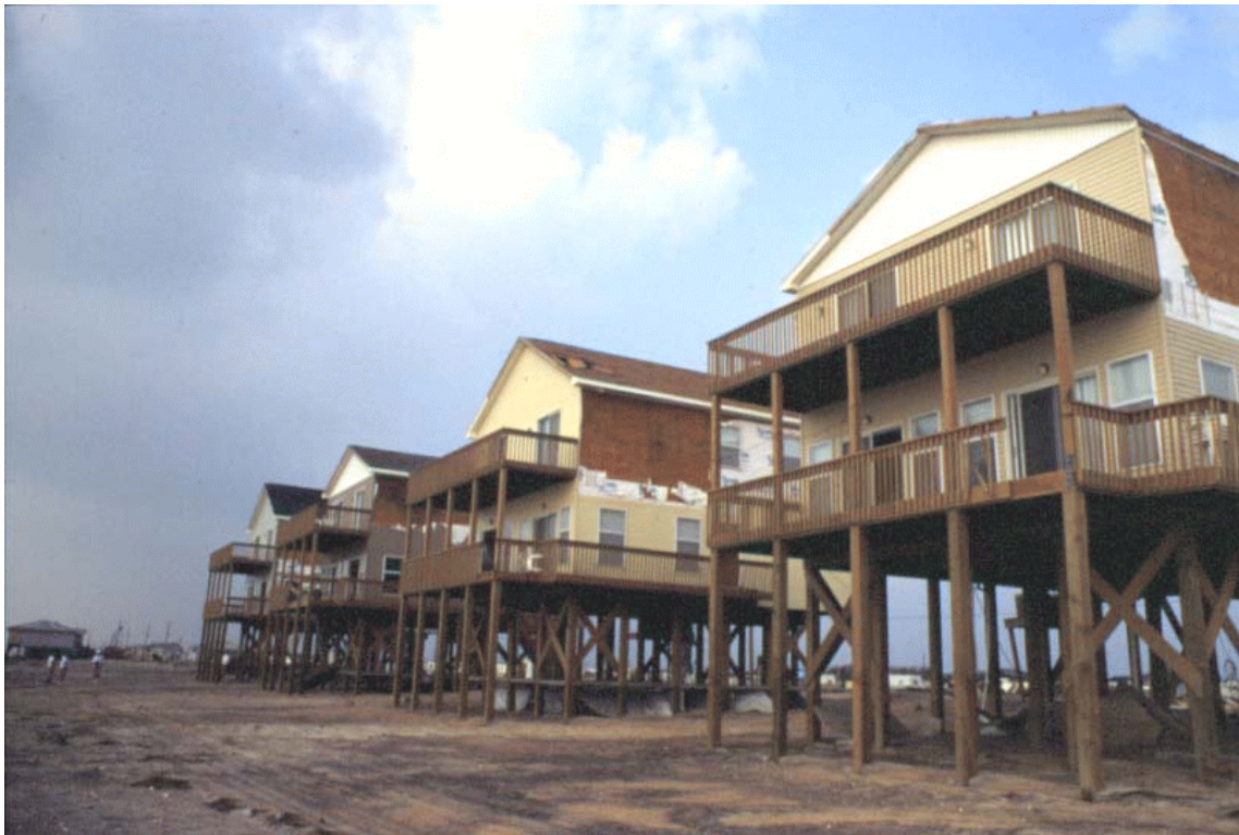
Figure 6: Houses on 1996 pilings (Class 1c) on low-elevation shoreline (Type B). Location: Topsail Island after Hurricane Fran.
