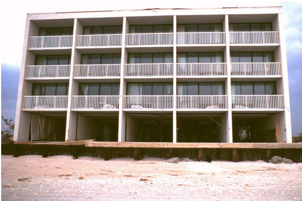
Figure 8: Piling-supported hotel with lower floor on unsupported slab (Class 2b) on low-elevation shoreline (Type B). Location: Wrightsville Beach NC after Hurricane Fran.
