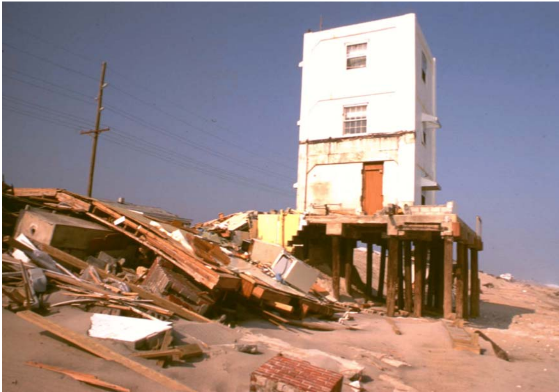
Figure 7: Slab foundation failure (Class 1a & 2a) beside commercial/deep-piling structure (Class 2c) on high-elevation shoreline (Type A). Location: Surf City NC after Hurricane Fran.
