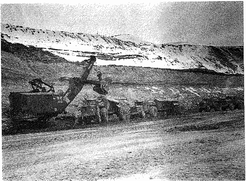
Power Shovel and Euclid Wagons Used in Excavation Operations for Powerhouse Area. December 1947.
