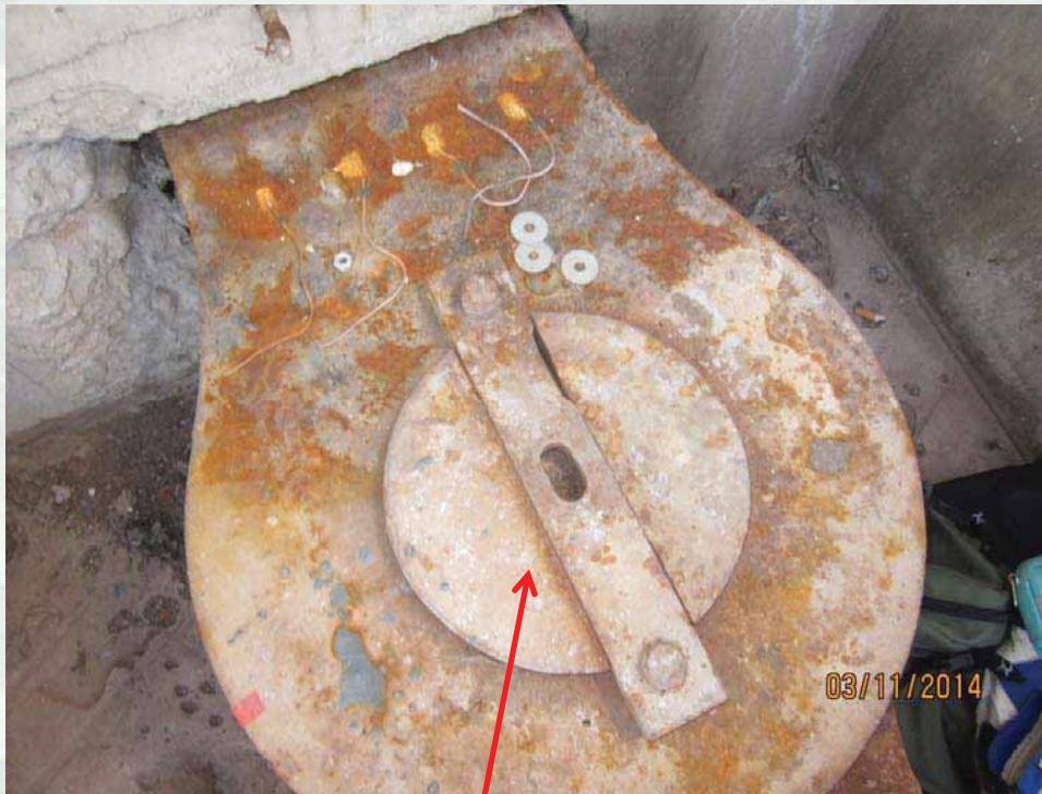
Gudgeon Pin to be replaced
