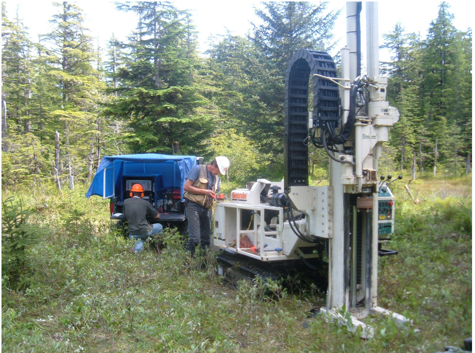
U.S. Army Corps of Engineers employees operate the Ultra Violet Optical Screening Tool (UVOST) and direct push drill rig during a remedial investigation at Yakutat in southeast Alaska.
