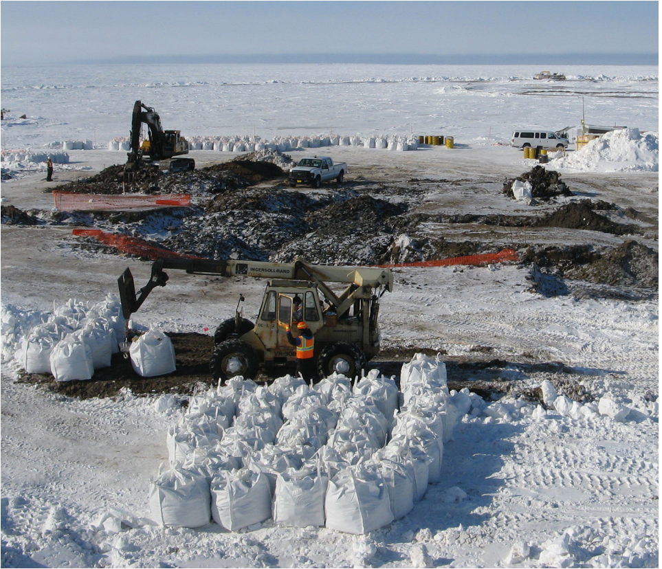
Contractors conduct contaminated soil excavation, containerization, and staging activities at the Air Force's Wainwright Long Range Radar Station on the remote northwest coast of Alaska. The project involved remote site logistics, barge transportation, and working in winter conditions.
