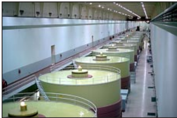
Generators in Chief Joseph Dam powerhouse, Columbia River
