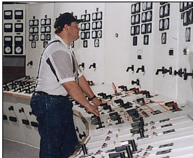
Control Room at Bonneville Dam, Columbia River
