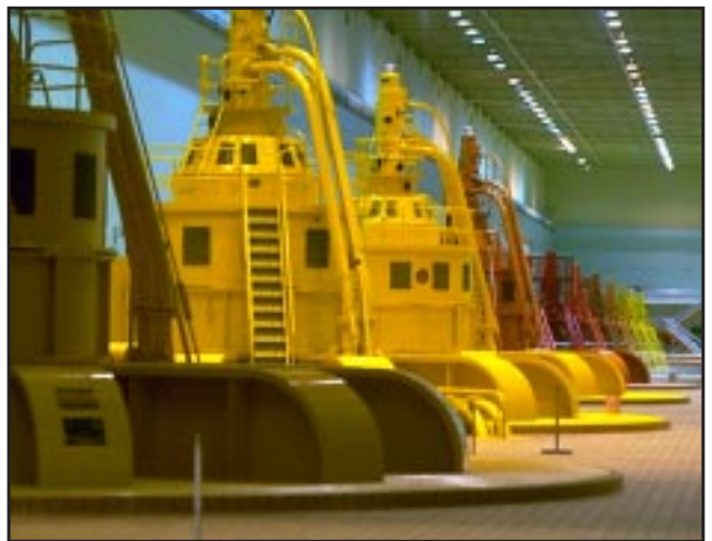
Generators at The Dalles Dam, Columbia River
