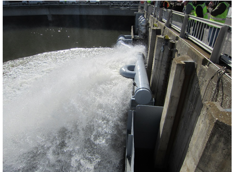
Semi-circular cool water spray at upstream end of Lower Granite Dam adult fish ladder. U.S. Army Corps of Engineers photo.
