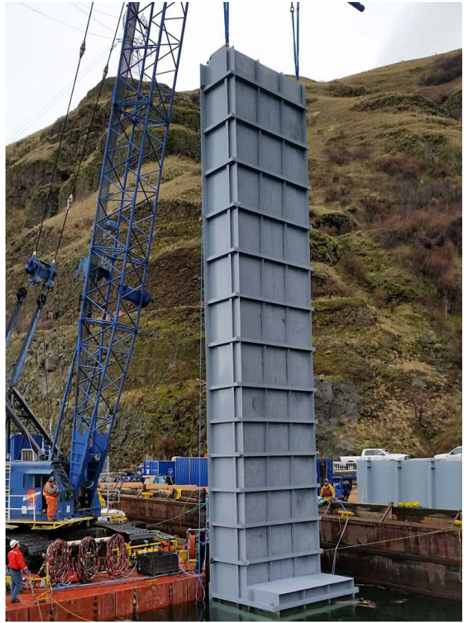
A supplemental water intake chimney provides supplemental water starting about 150 feet down from the top of the fish ladder, plus water to the adult fish trap. U.S. Army Corps of Engineers photo.
