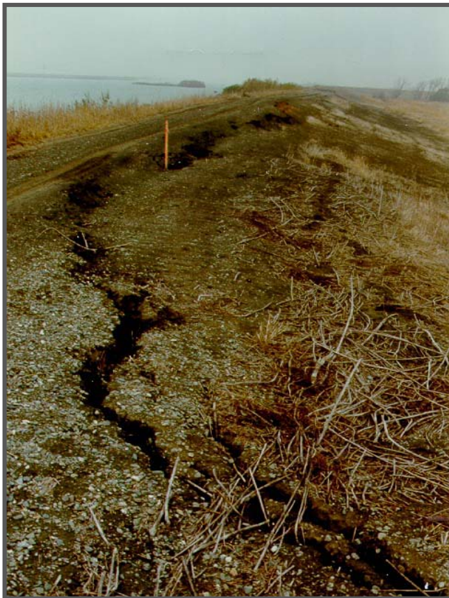
Figure 2-4. Slope Stability Failure on the Natomas Levee during the 1986 Flood.
