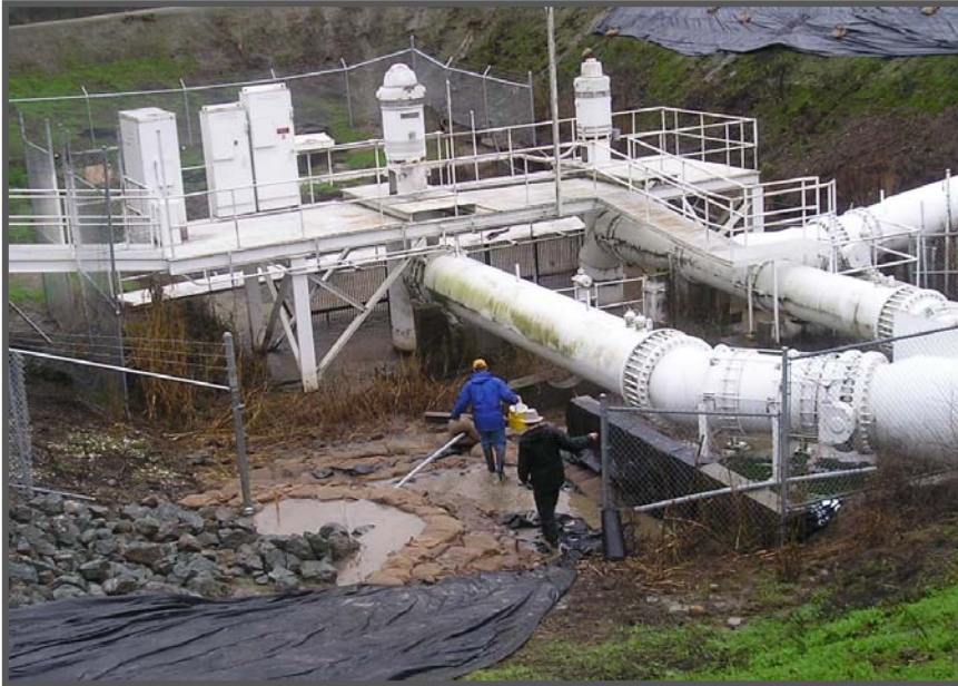
Figure 2-5. Sandbag Ring on Sand Boil on the Natomas Levee during the 2006 Flood.
