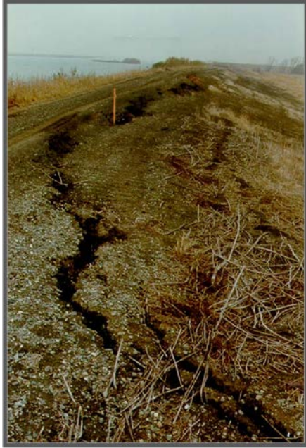
Figure 2-4: Slope Stability Failure on the Natomas Levee during the 1986 Flood.
