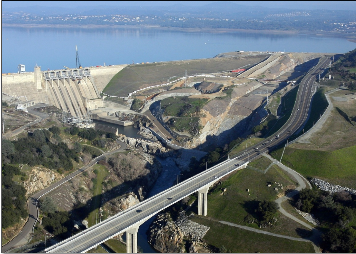
Figure 2-12: Construction in Progress at Folsom Dam as part of the Folsom JFP.
