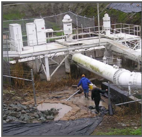
Figure 2-3: Sandbag Ring Surrounds a Sand Boil on the Natomas Levee during the 2006 Flood.
