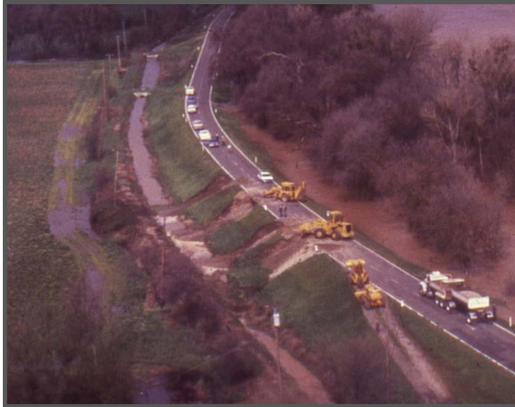
Figure 2-1: Slope Failures on the Landslide of the Levee and Seepage Exiting at the Levee Toe on the Garden Highway in Natomas during the 1986 Flood.
