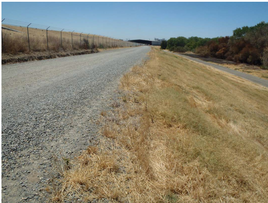
HTRW FIGURE 18 -ARS Reach B (5)/C Sacramento City Landfill rises above levee crown in the left side of the photo. Stormwater collection drain is visible. Landfill gas collection system is obscured by the weeds.
