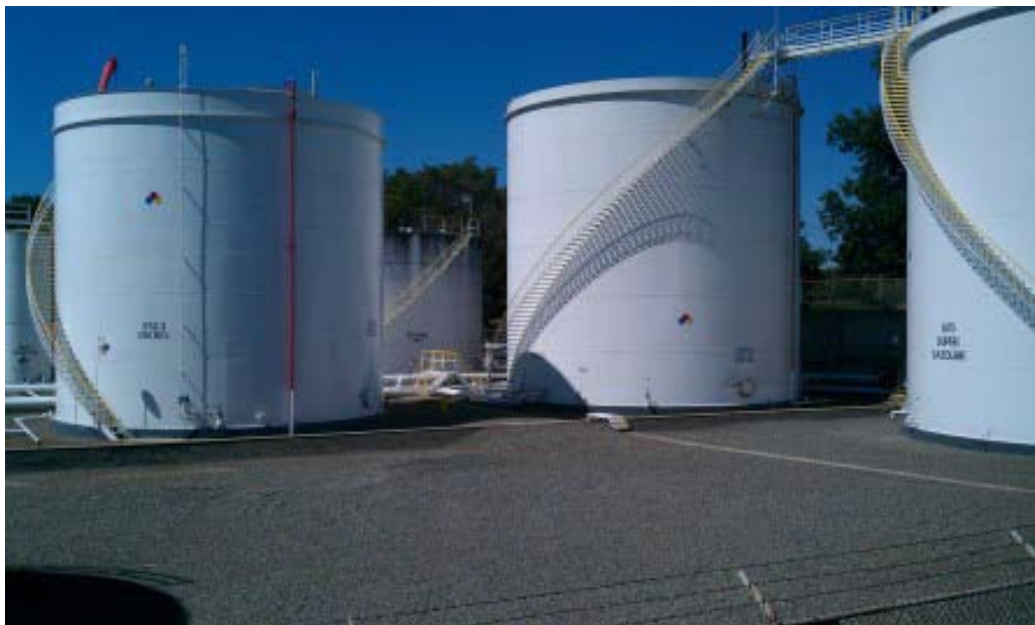
HTRW FIGURE 22 - ARS Reach D 76 Broadway (4) is a bulk fuel terminal used by Conoco Phillips. Underground infrastructure and at least 7 above ground storage tanks containing petroleum substances are located on both sides of the levee.
