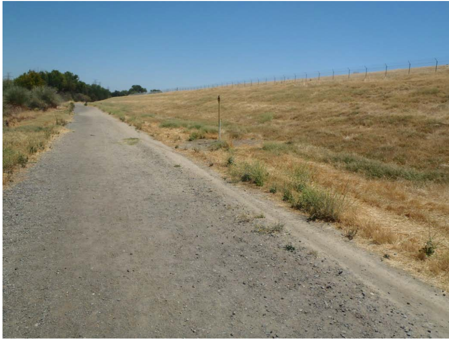
HTRW FIGURE 17 - ARS Reach B(5) Kinder Morgan Energy Partners buried petroleum pipeline warning sign at the toe of the levee at Sacramento City Landfill /Sutter Landing Regional Park
