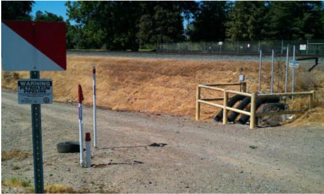
HTRW FIGURE 23- ARS Reach D (4) Fuel lines cross through the levee at 76 Broadway.
