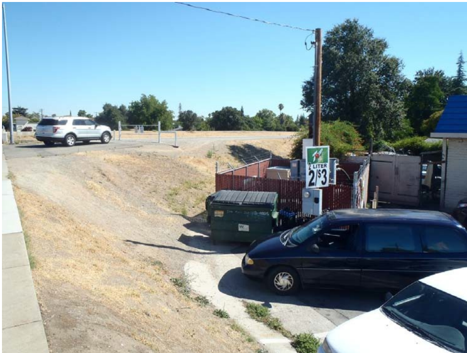
HTRW FIGURE 12 -ARN Reach N (2) Full Stop Mini-Mart SVE/AS treatment system located adjacent to levee
