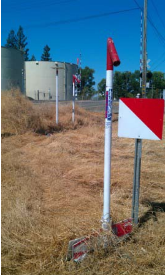
HTRW FIGURE 25- ARS Reach D (3&4) Fuel lines cross to and from the water and land sides of the levee to the following sites: 76 Broadway (ConocoPhillips Bulk Fuel Terminal), 66 Broadway (TOSCO Corp Sacramento Terminal), and 2420 Front St (Chevron Bulk Fuel Terminal).
