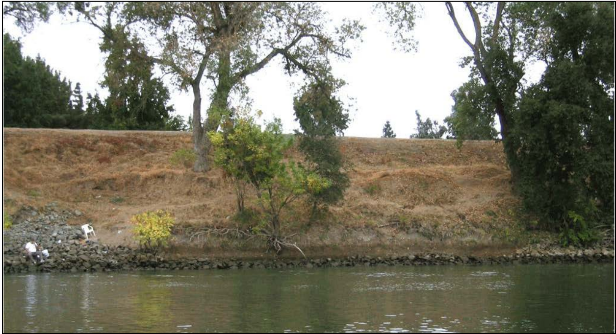
Figure 2-6. Erosion site of the left bank of the Sacramento River at RM 53.2 (2005)
