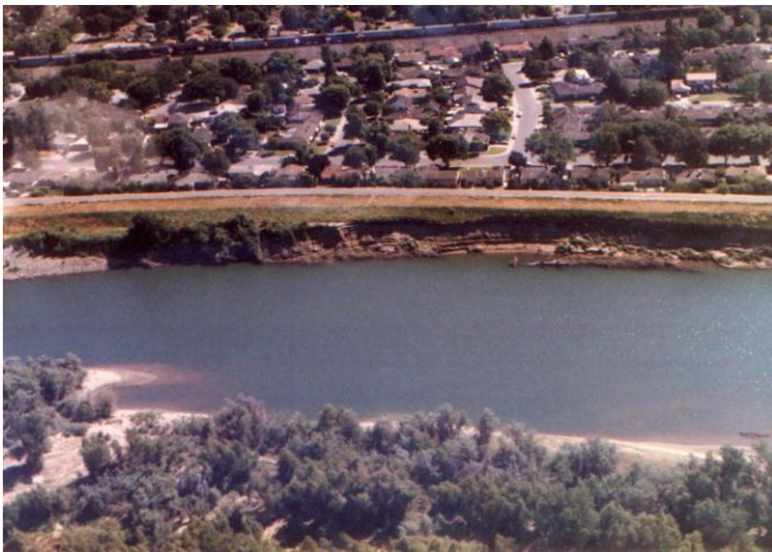
Figure 4-1: 1986 Erosion Distress on the American River South Bank Near I-80
